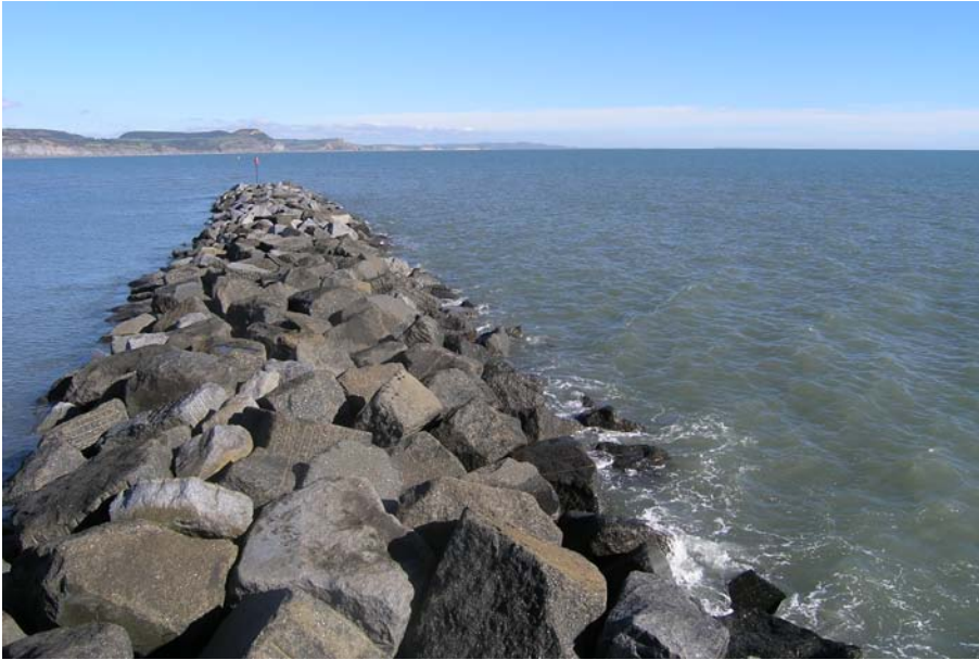
Plate 4: View along rock armour at end of South Arm of the Cobb.
