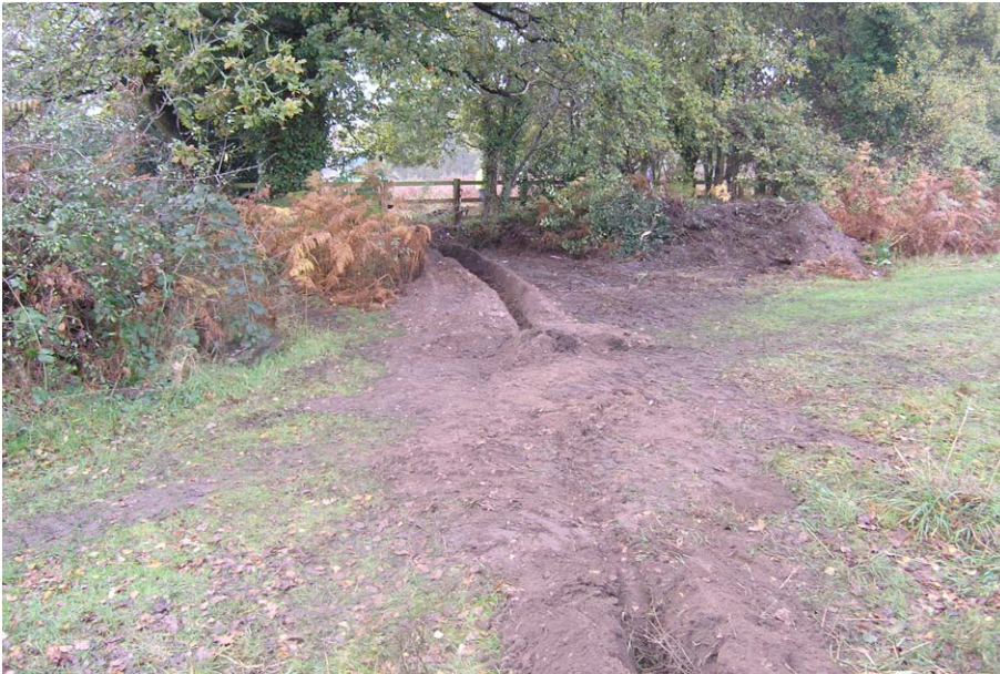
Plate 1: View of northern part of the central section of the pipe trench.
