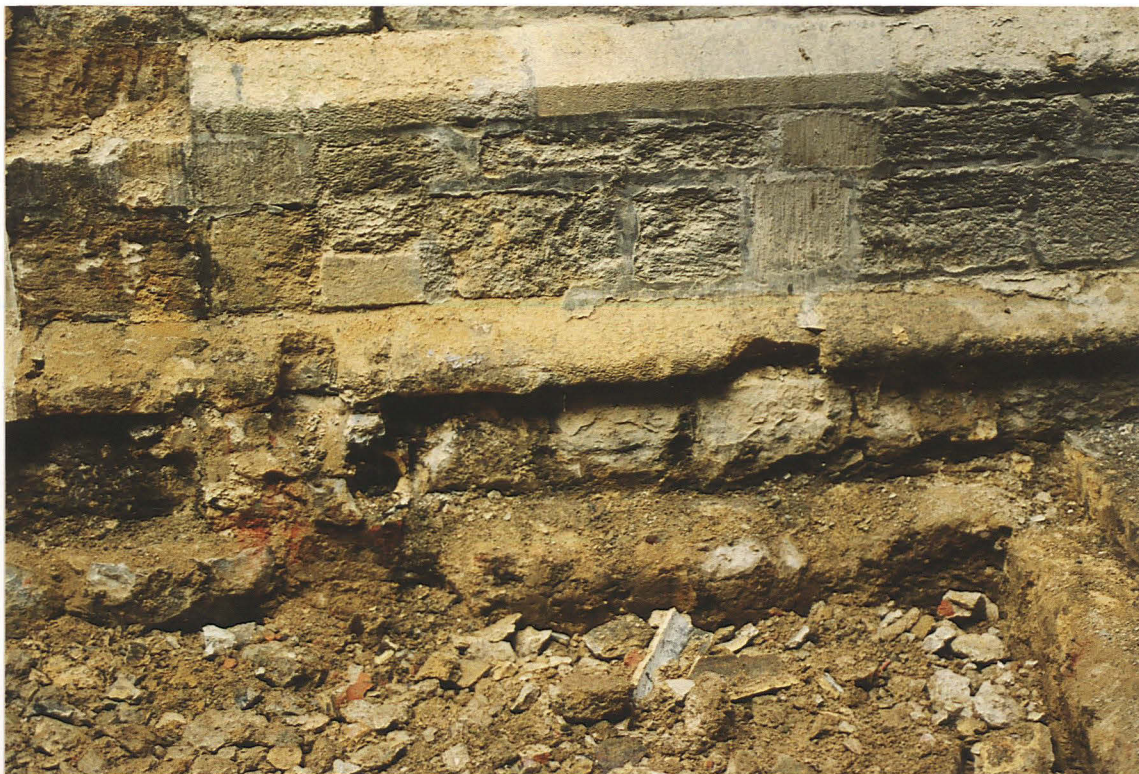
Pl. 8 Foundation to north wall of St Thomas' Chapel, looking south-west, with foundation of south transept showing to the right.
