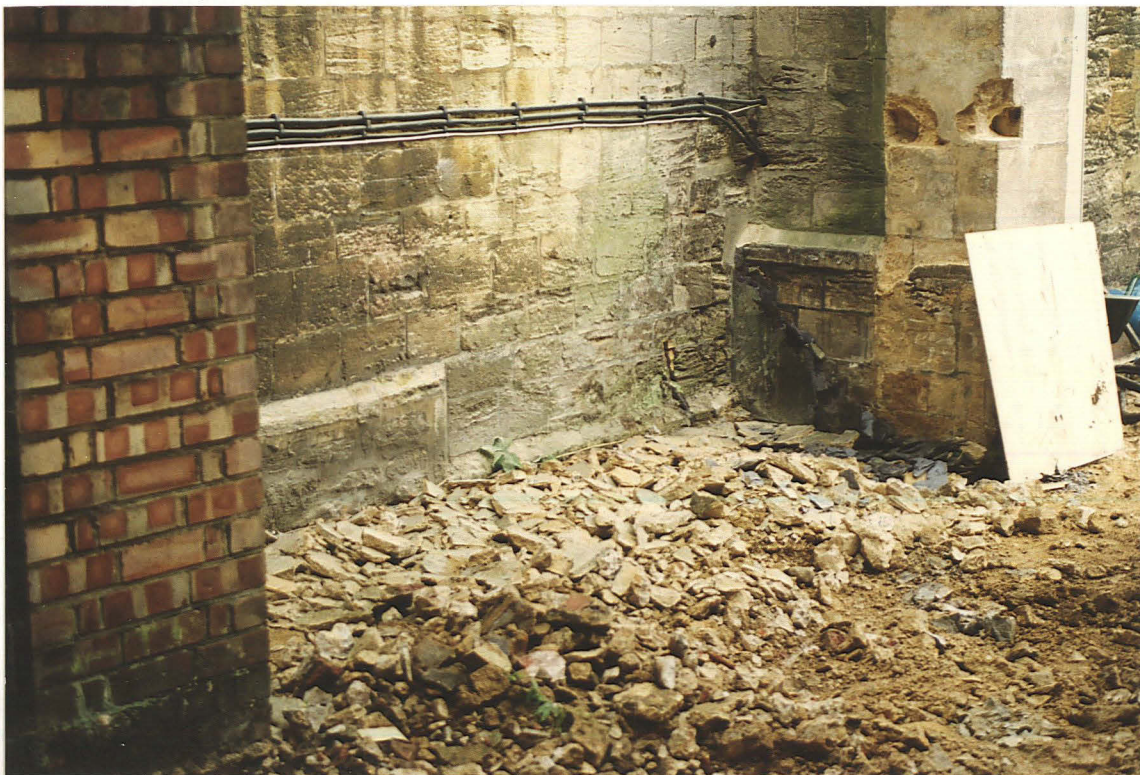
Pl. 2 South wall of chancel, looking north-east. The demolished passageway butted up against the buttress to the right of the photograph.
