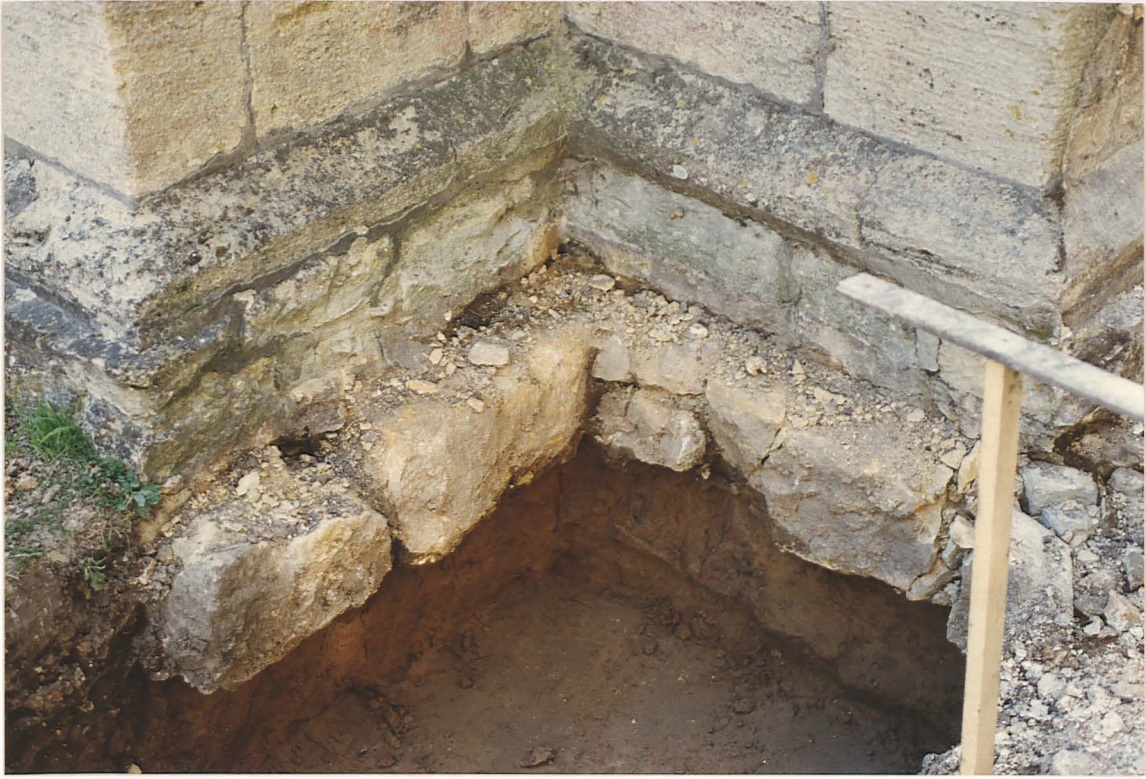
Pl. 5 Foundation of the buttress on the north-east corner of St Thomas' Chapel, looking south-west.
