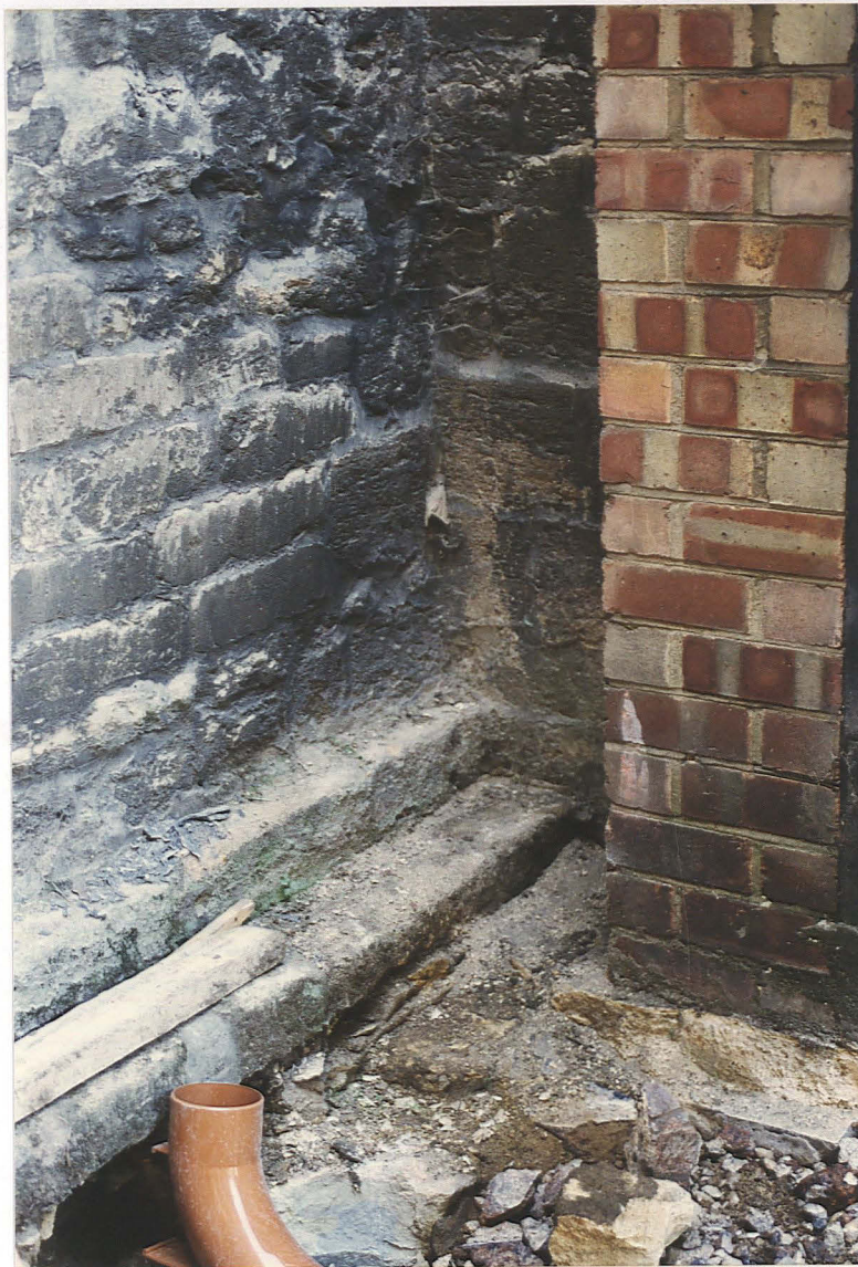
Pl. 7 Corner of south transept and chancel wall, looking north-west, with housing for organ bellows on the right, showing contrast in foundations.
