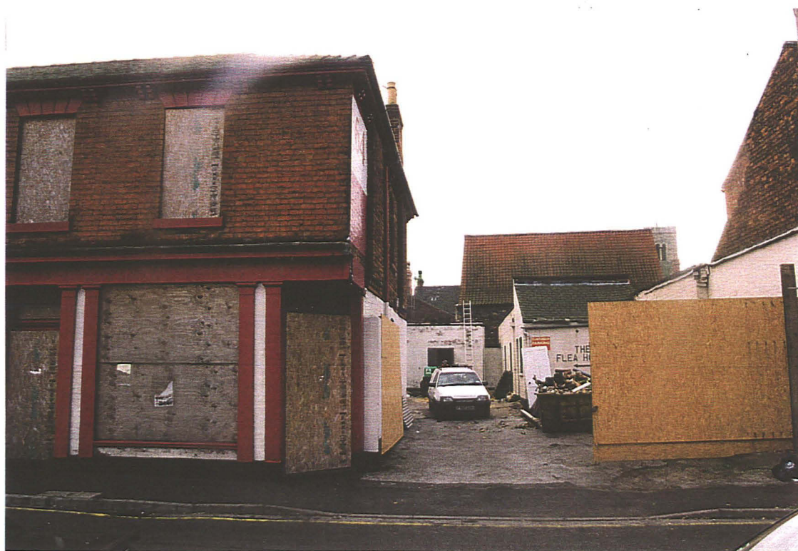
Pl.1: A general view of the existing buildings at 64 Monson Street prior to the commencement of work. The nineteenth century brick shop frontage in the foreground was retained for conversion and the other buildings visible in the yard have been demolished. St. Mary's Guildhall (with the pan-tiled roof) and the tower of St. Peter-at-Gowts' church are visible to the south of the site.
