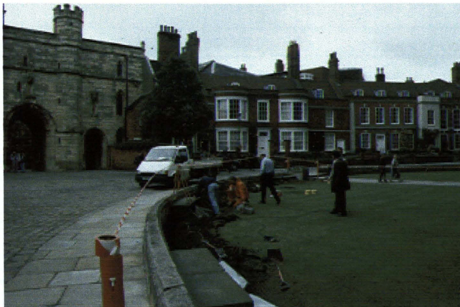
Plate 1 - View of the Cable Trench, at the west end of the Cathedral
