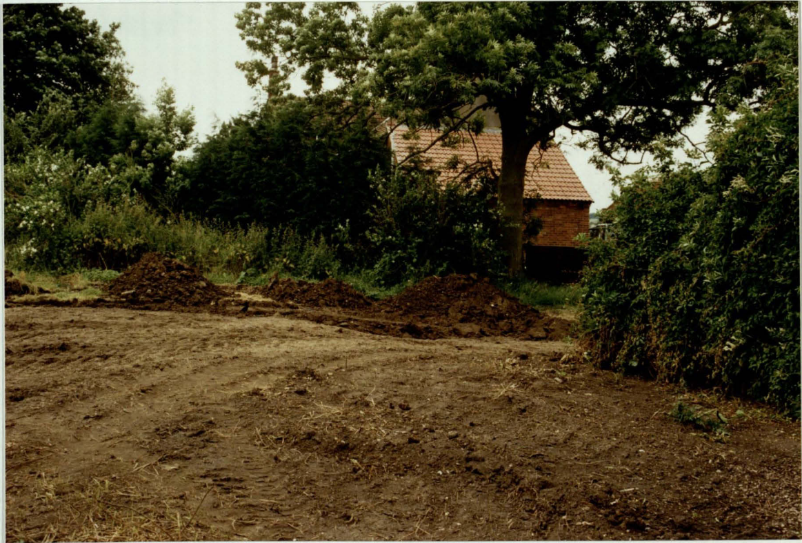
Pl. 4 The depression visible east of the lane to The Farm. The trench excavated for the new sewer is visible (looking south).
