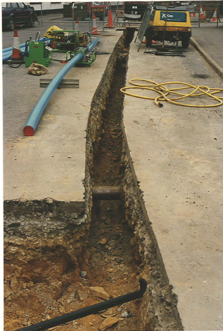
PI. 8 High St, view looking north from the Market Cross (observation 14), showing numerous services crossing the pipe trench
