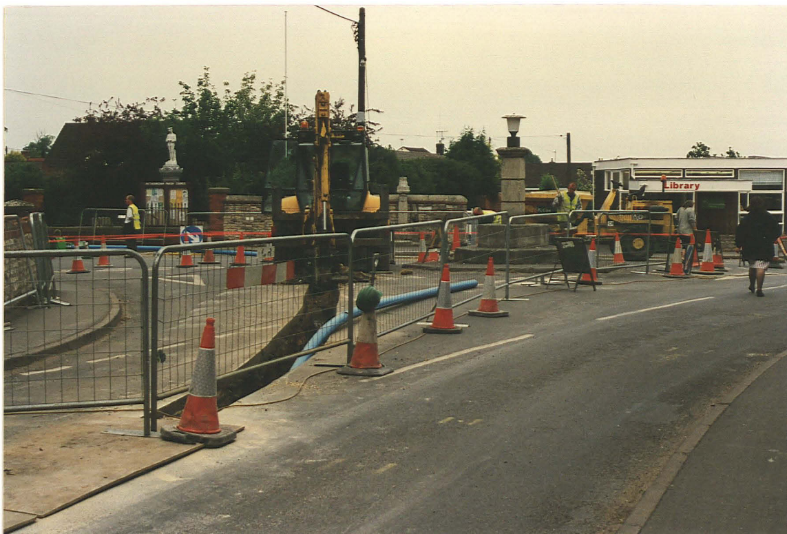
Pl. 4 Junction of Prince's St and High St, looking east. Note medieval cross to right of JCB
