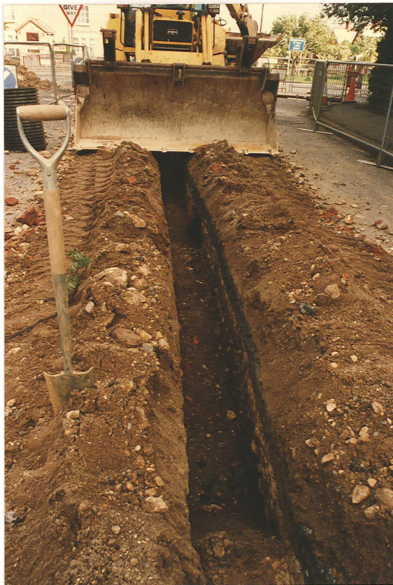
Pl. 5 North end of High St, looking north, showing brick culvert , observation 10, just below machine bucket.
