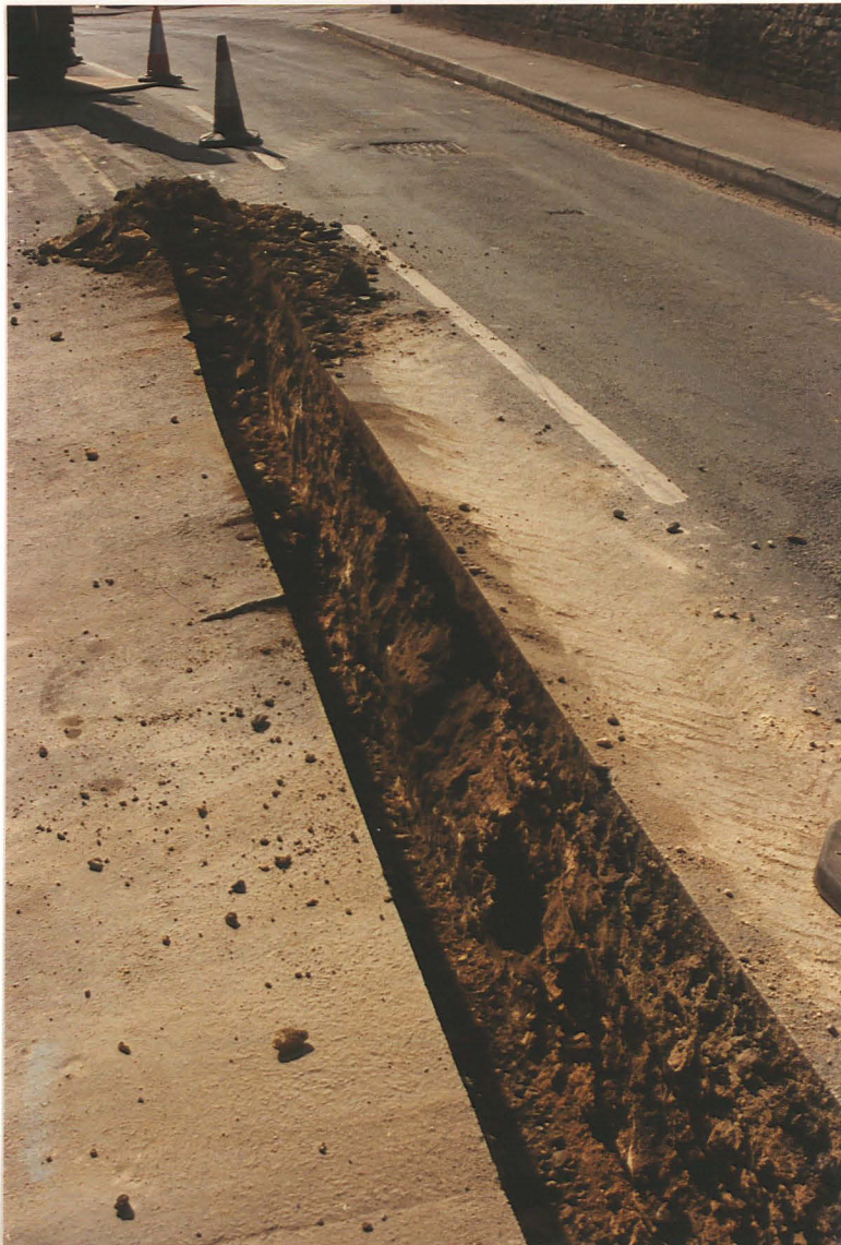
Pl. 13 High St, observation 16, opposite old school, showing small ditch or pit on right hand side of trench, filled with grey-brown clay, looking south.
