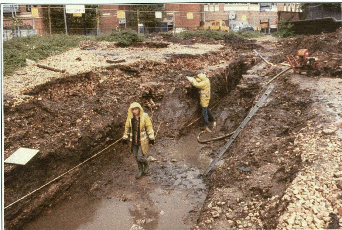
Plate IV: Trench 3, looking east south-east. As the base of the trench lay below water level, water was a constant problem (note the pump). Reclamation deposits, dipping towards Brayford Pool, can clearly be seen in the lower left-hand corner of the photograph.
