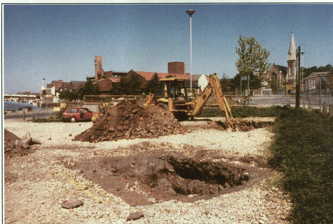
Plate 1: General view of the site looking west north-west showing the machine excavation of Trench 2 (Trench 1 can be seen in the foreground).
