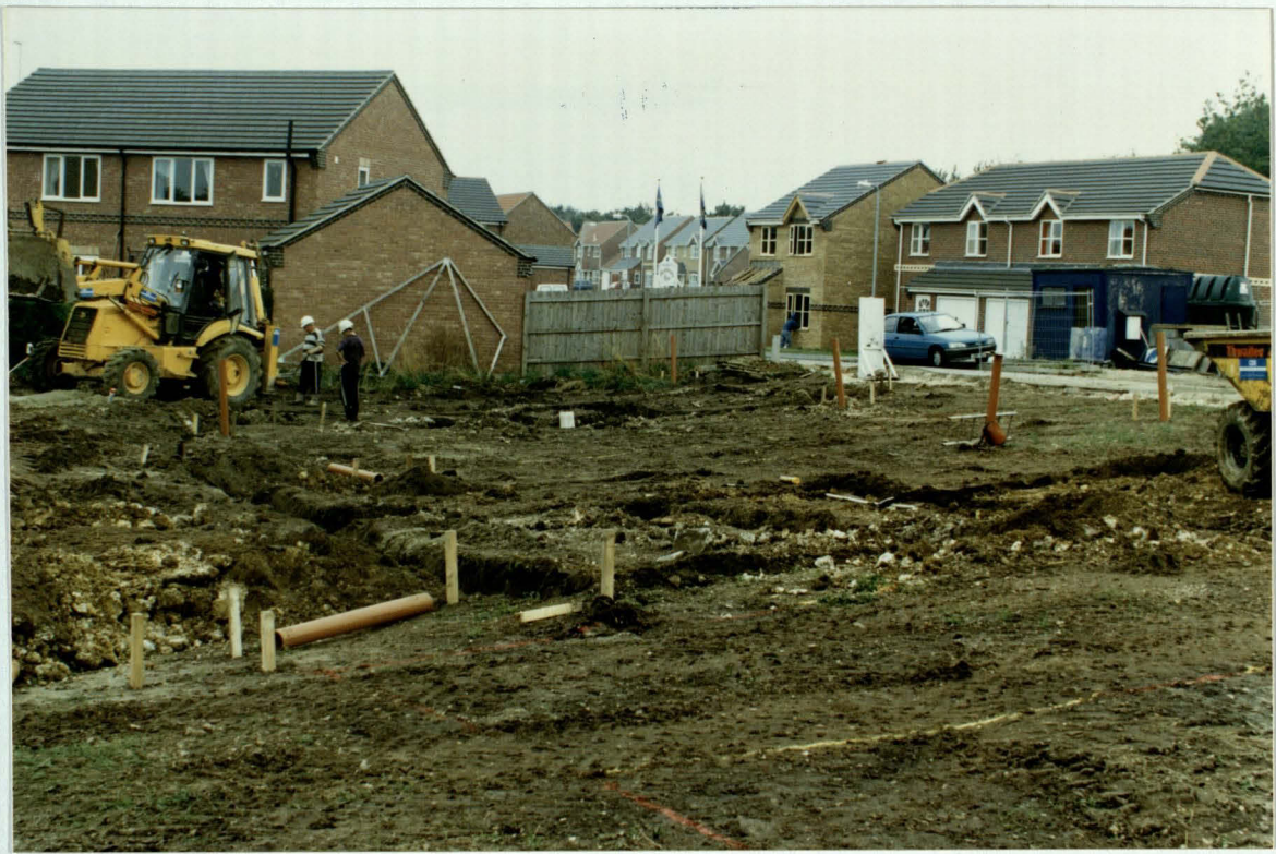
PI. 5 Foundation trenches for Plot 5 S (foreground) and Plot 54 (by machine). Looking south.
