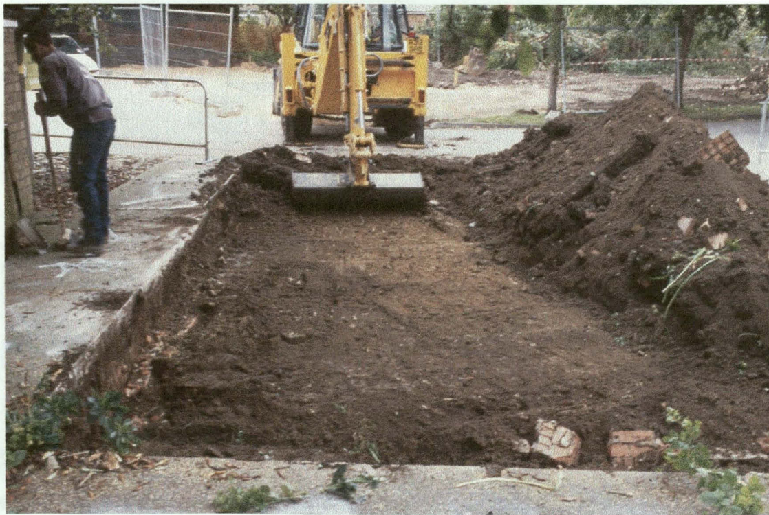
Plate 2: Excavation in progress for the access road to the west of Church View (looking north/ north-east).
