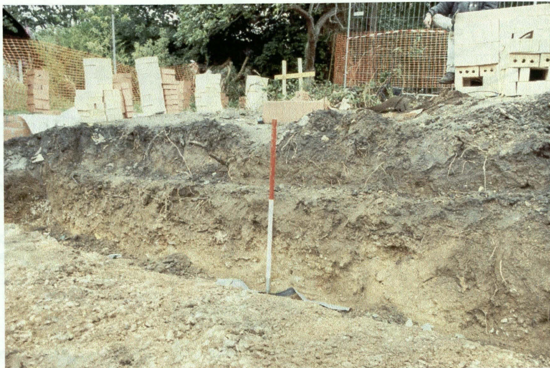
Plate 3: General view of work in progress over the extension plot area (looking south-east)
