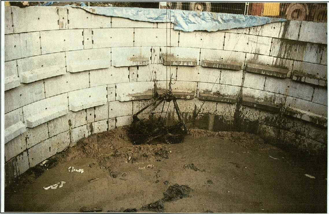
Plate 1: View of excavation for main pumping chamber (Area 1) in progress, showing methodology
