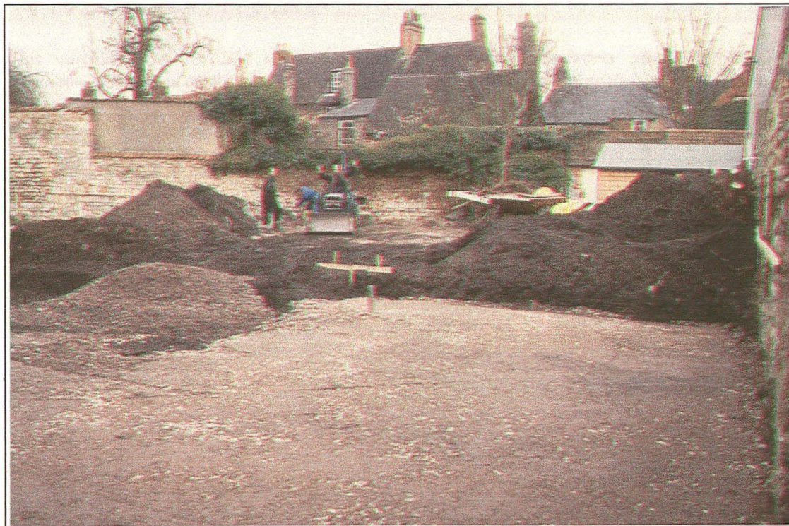
Plate 1: General view of the site, looking east, during the reduction of ground level, prior to the casting of the floor slab.
