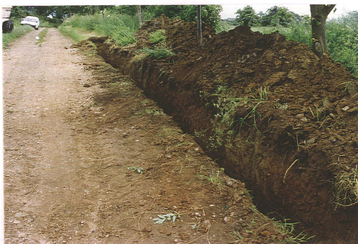
Pl. 9 The pipe trench was sited in the southern verge of the track. A thick root (right foreground) is above ditch 1E.
