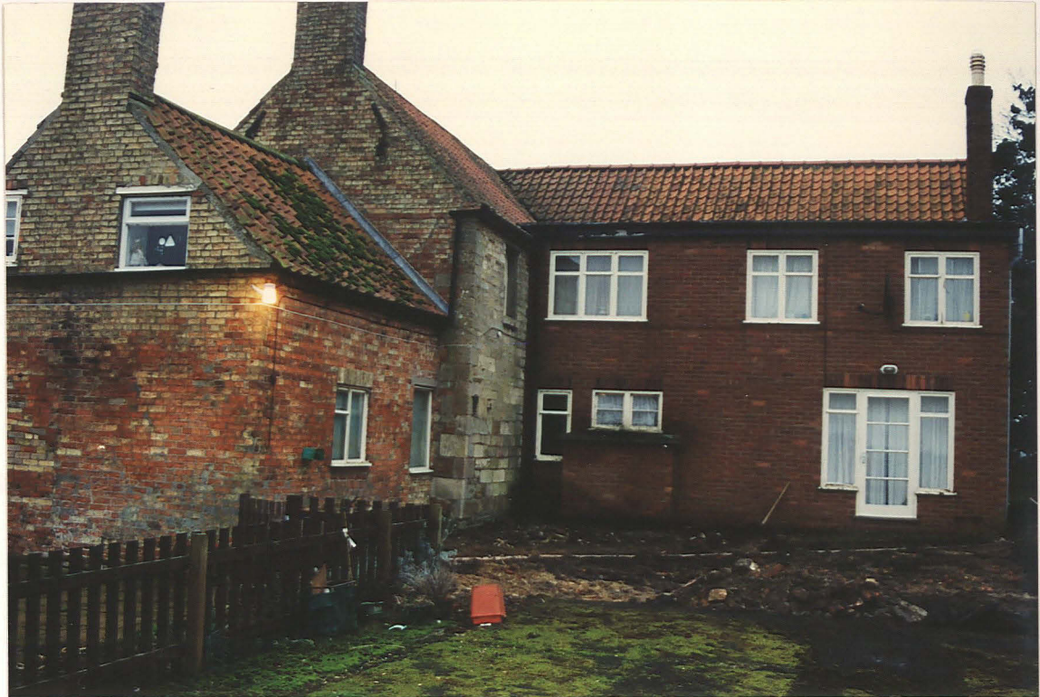
Pl. 2 Position of the new extension, after removal of the tennis court surface. Looking SW.
