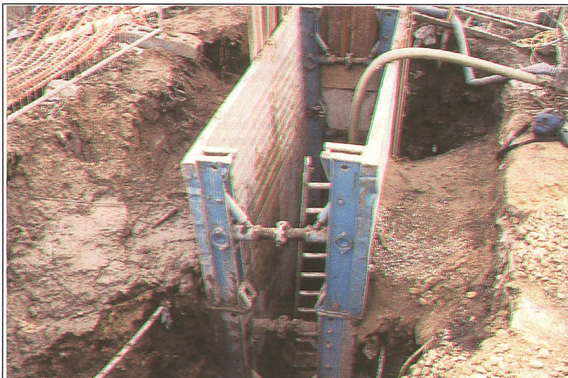
Plate II: General view of main drainage connection works. The depth of the trench required the insertion of box-shoring, severely restricting the amount of recording possible.
