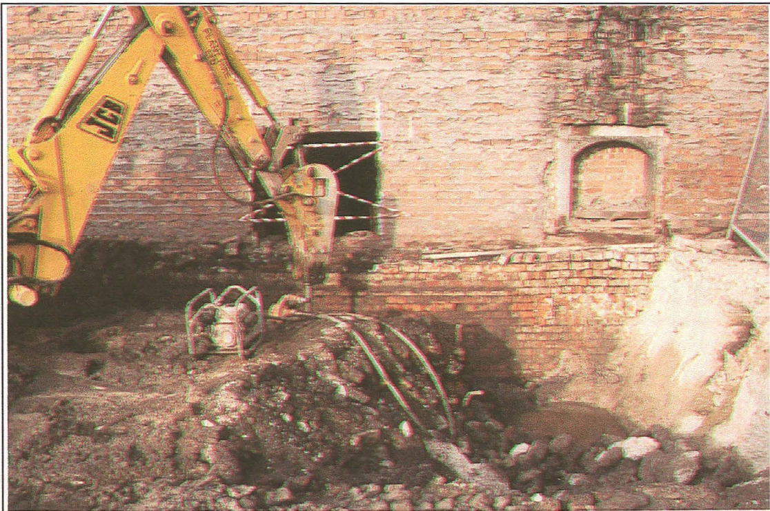
Plate I: View looking north, showing the excavation for the removal of buried obstructions (in this area concrete up to 1.80m thick was encountered) to the south of Building One. Previous remodelling to the mill buildings had severely disturbed archaeological deposits across much of the site.
