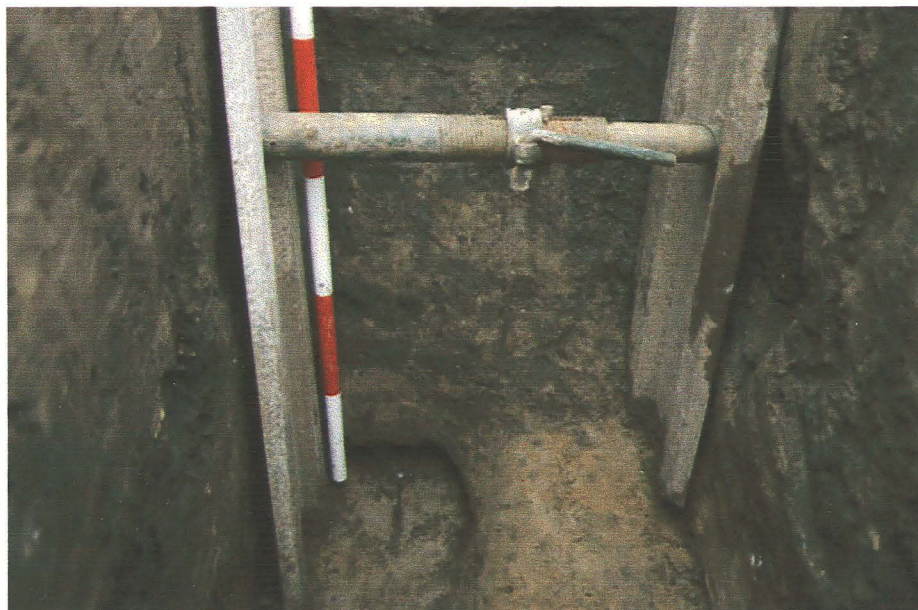
Plate 2 - Section 2 and the base of the pipeline trench showing the cut for the grave, looking north
