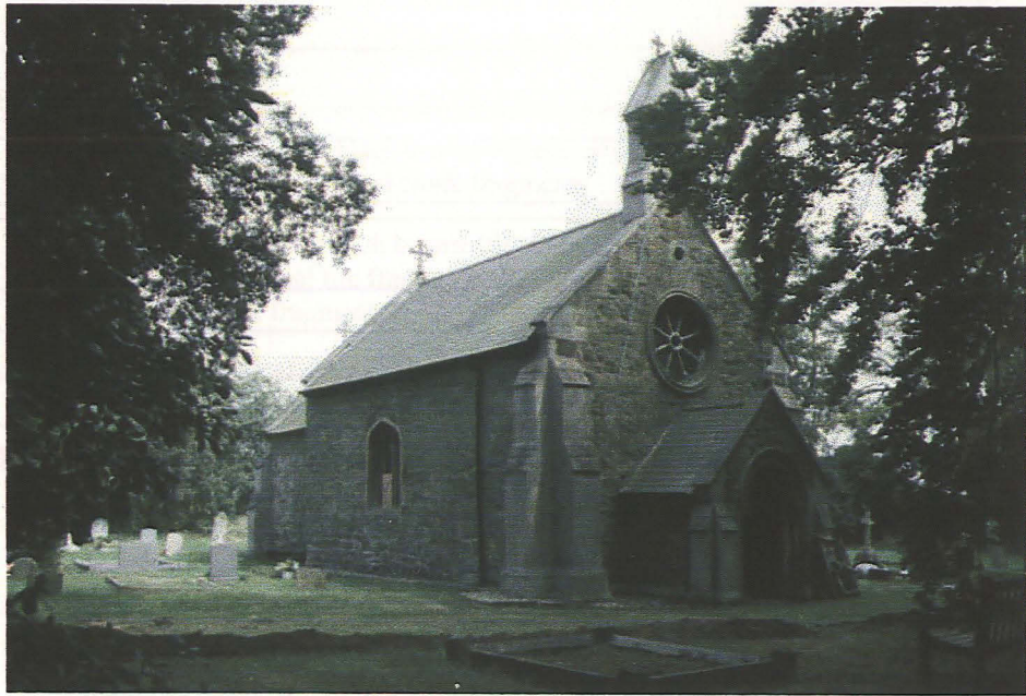
Plate 1 - St. Andrew's Church, with the pipeline trench in the foreground, looking southeast
