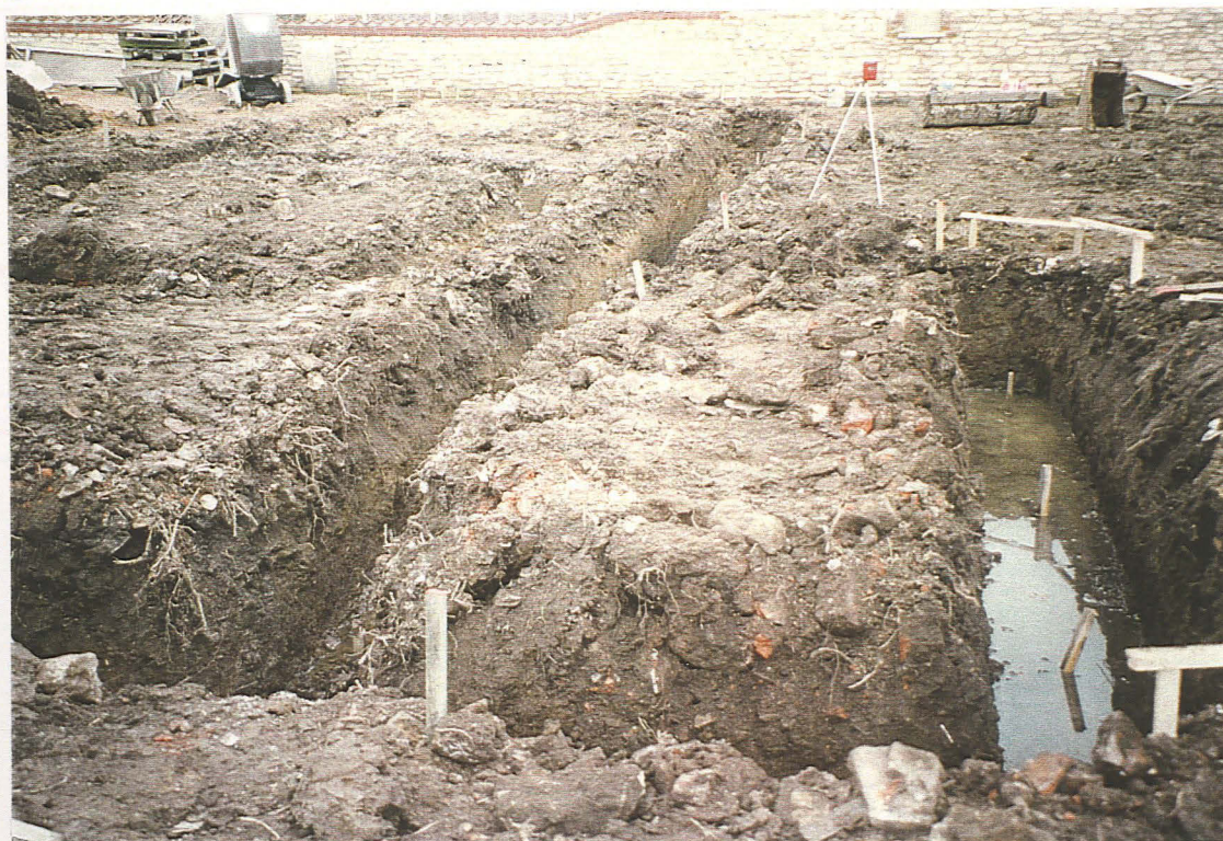
P.2 General view of house foundation trenches looking west, showing rubble from demolished agricultural buildings.
