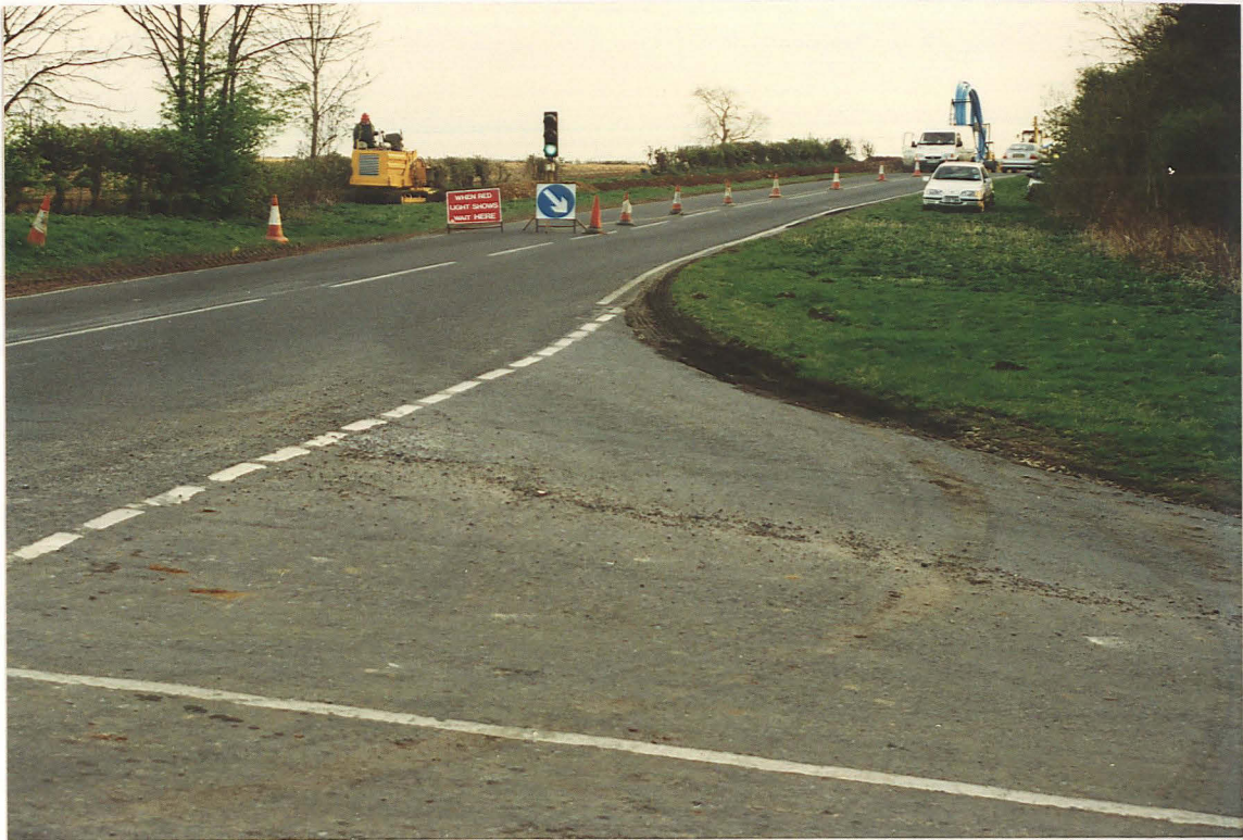
Pl. 1 Trenching for the replacement main, south of the Pottergate Road junction near The Mill Farm (looking south).
