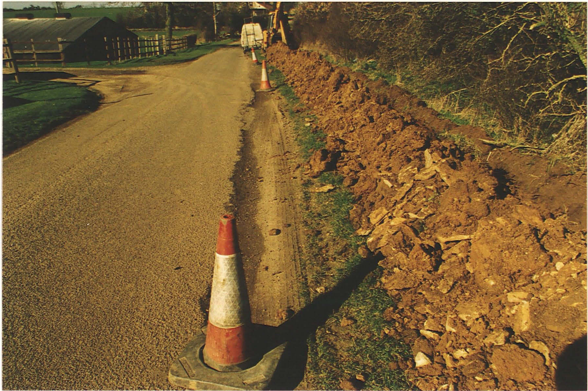
Pl. 3 Limestone pieces in the trench spoil, interpreted as post-medieval consolidation of a former watercourse.
