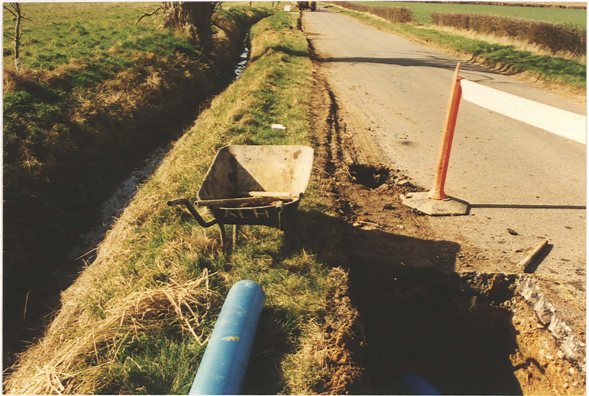
Pl. 8 Position of Trench 3, Lenton-Pickworth Road. The JCB is beside the footpath; the Roman road is thought to cross between these points (looking SW).
