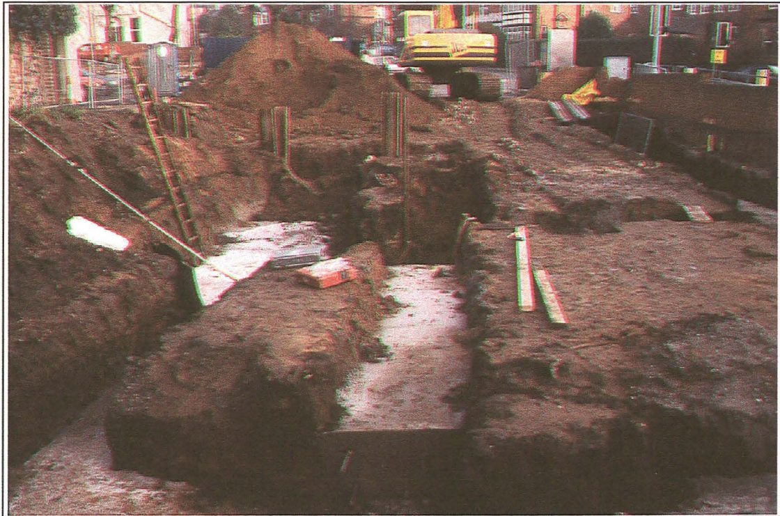
Plate 1: General view looking north-east across the site during the excavation of the foundation trenches. Although extensive, the foundation trenches were thought to have disturbed no important archaeological remains.
