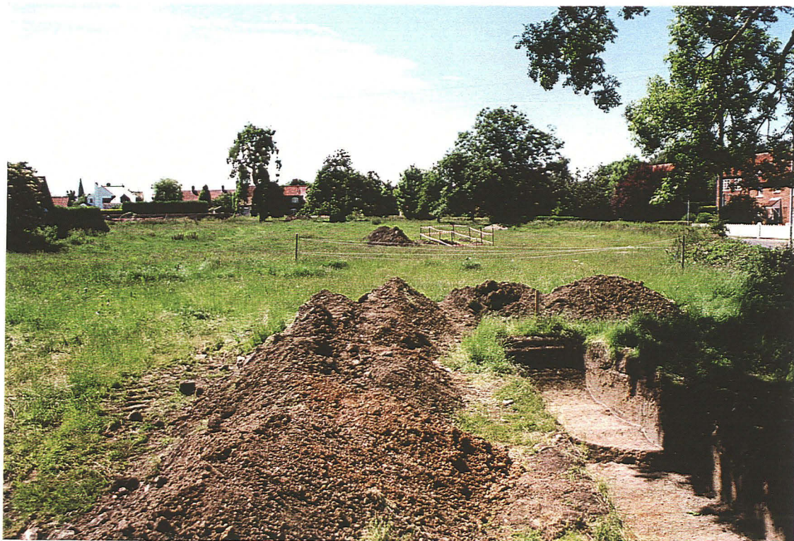
P.1 General view of the site with Trench 1 in the foreground, looking west.
