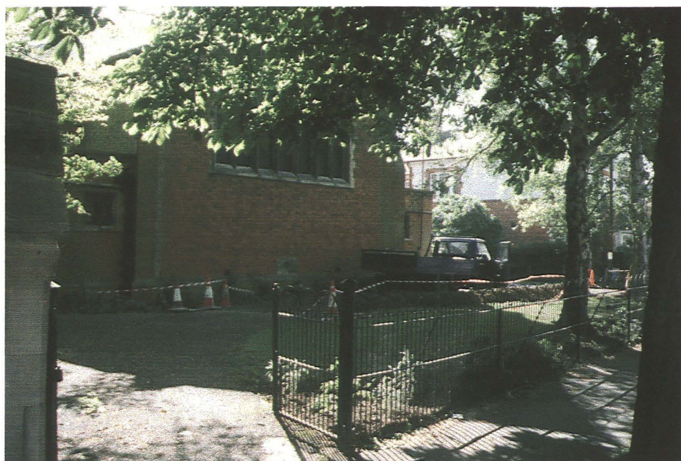
Plate 1 General view of St. Anne's church, showing the excavation of the service trench, looking southeast
