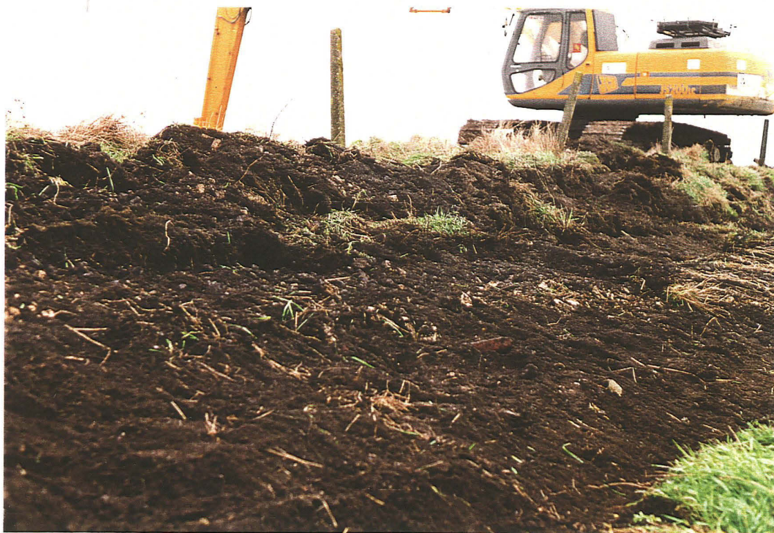
P.2 General view of the topsoil strip for the reprofiling of the embankment, looking west.
