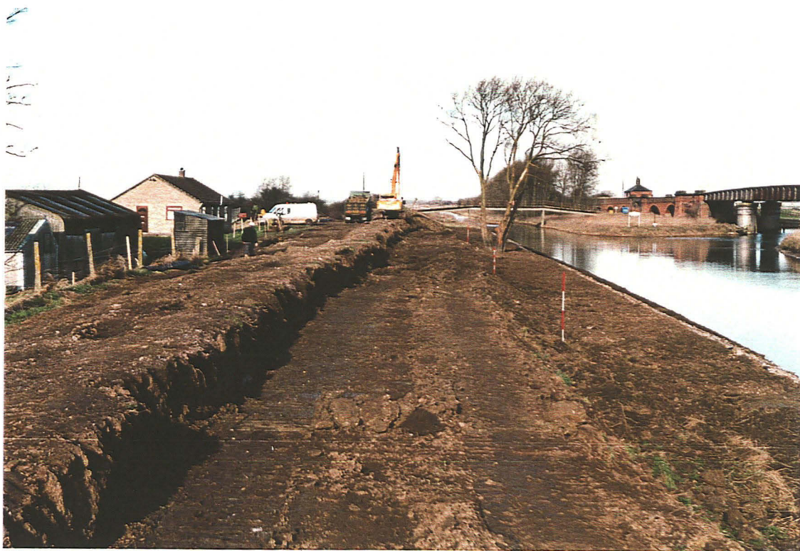
P.1 General view of the stabilisation of the Witham bank and the excavations into the upper portion of the embankment, looking north-east.
