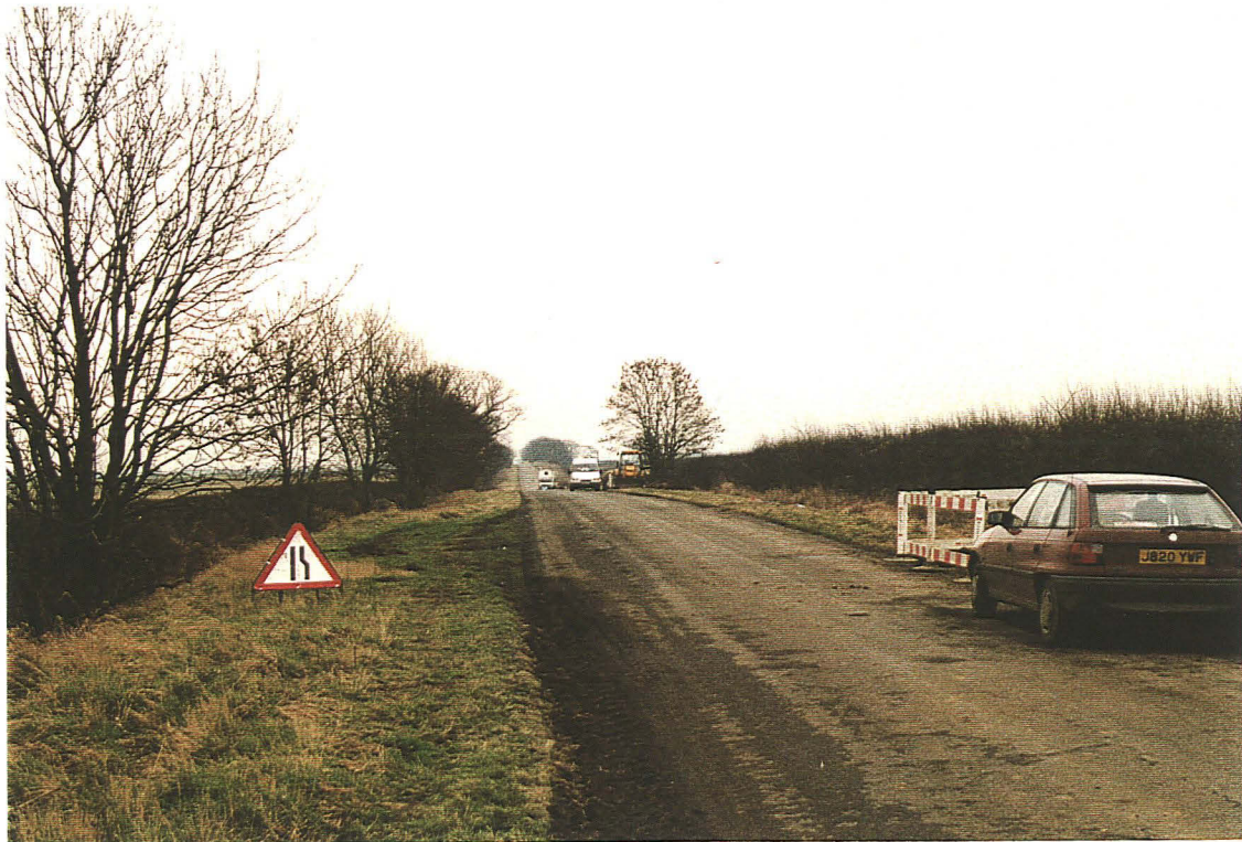
P.1 General view of mains replacement in progress on Ermine Street (area 2), looking south.
