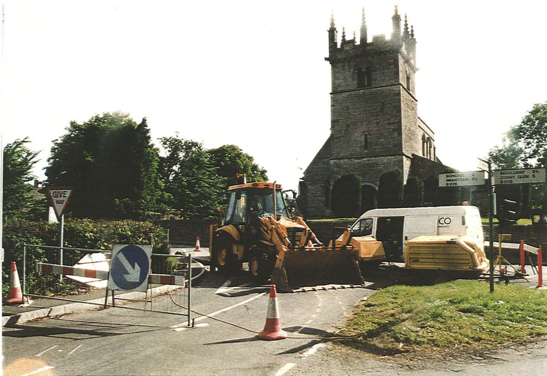
P.1 General working shot of the mains replacement in area 1, looking east.
