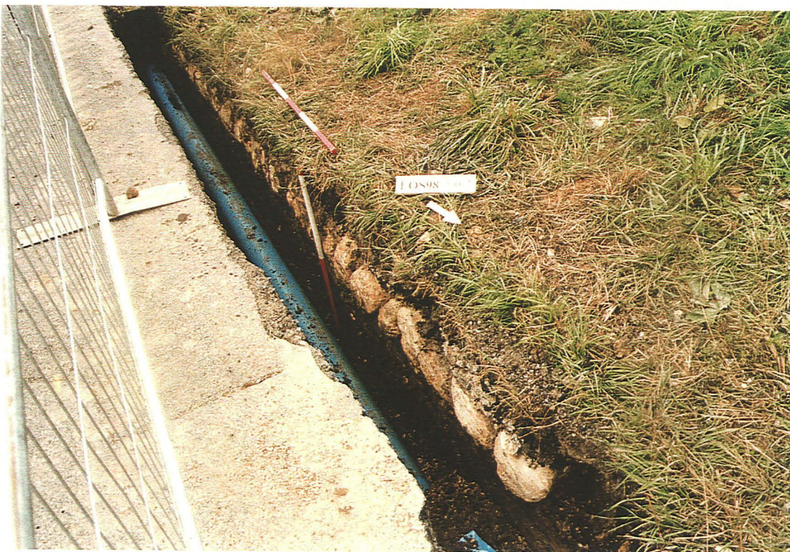
P.2 General shot of pipe trench in area 1 showing stone structure [102], looking south-west.
