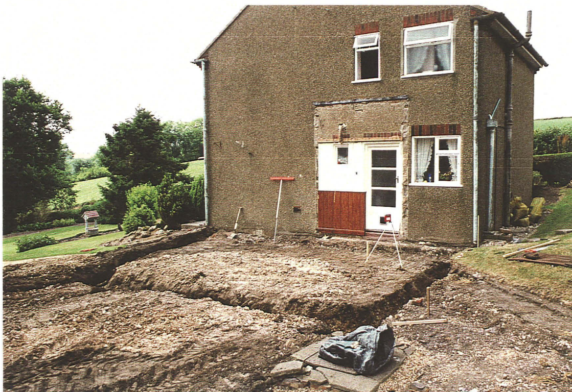
P.1 General view of the foundation trench for the extension, looking west.
