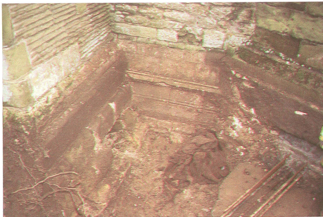
Plate 2: View of interface between original tower masonry (centre), 15 th century buttress (left), and 1886 buttress (right) on north side of tower - looking south
