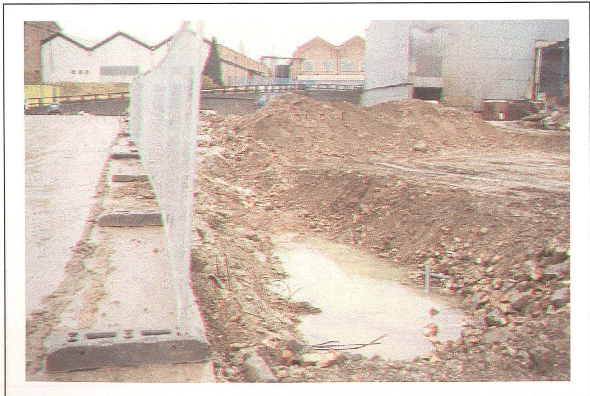
Plate 2: View of excavated area, central part of the site, showing modern intrusive material - looking east
