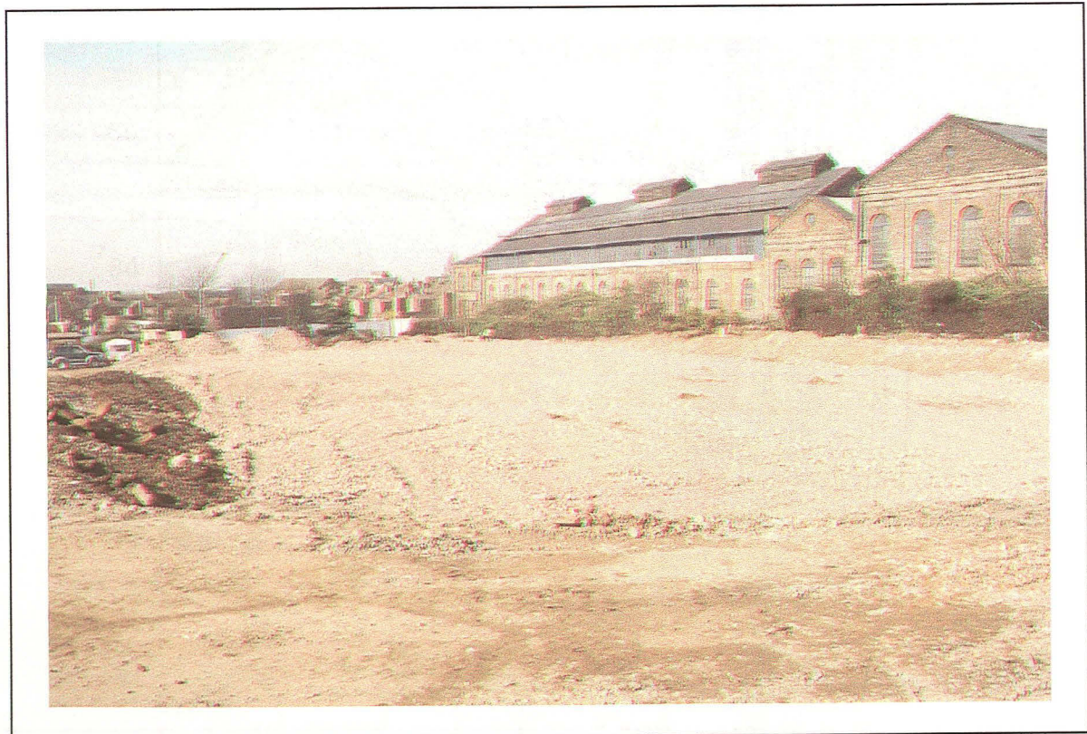
Plate 4: View of hardcore 'piling mat', in advance of piling operations, main store area - looking north-west
