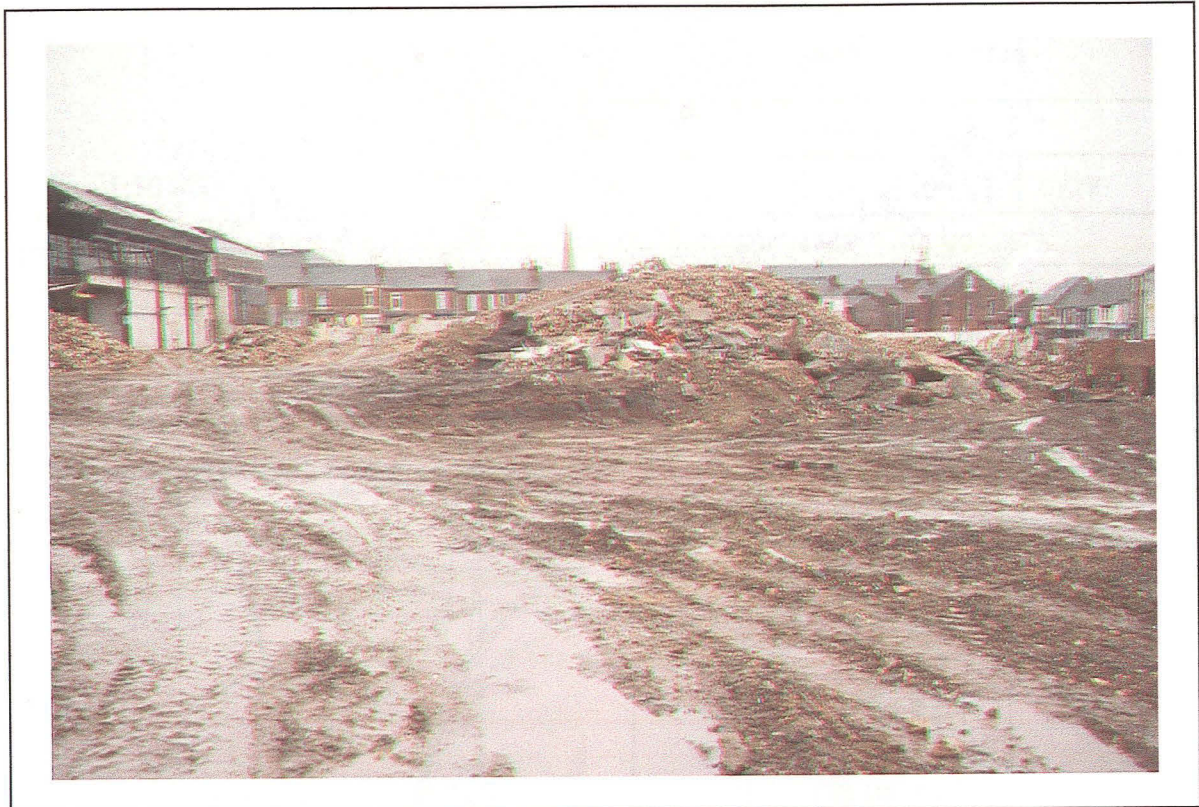
Plate 3: View of site following demolition of majority of former engineering works - looking south
