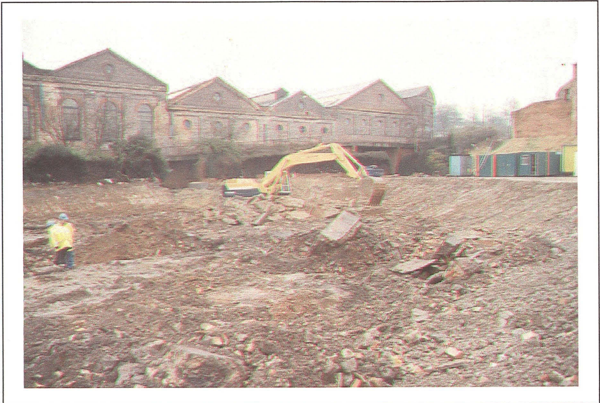
Plate 1: General view of site stripping/level reduction groundworks underway at the northern end of the site - looking north-east
