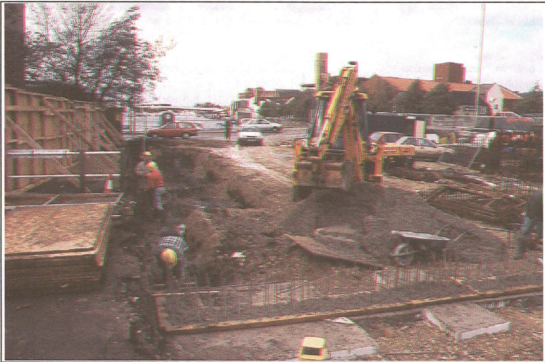
Plate 1: General view of the site, looking west as the development's groundwork progresses. Although apparently destructive, mitigation measures have ensured that much of the buried archaeological resource has been preserved in situ.
