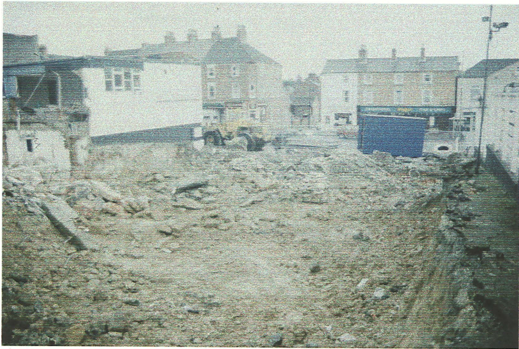
Plate 1 General view of site, looking east. Section 1 is located on the right.
