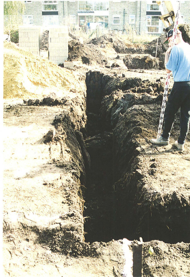
P.4 General view of footing showing section collapse, looking east.
