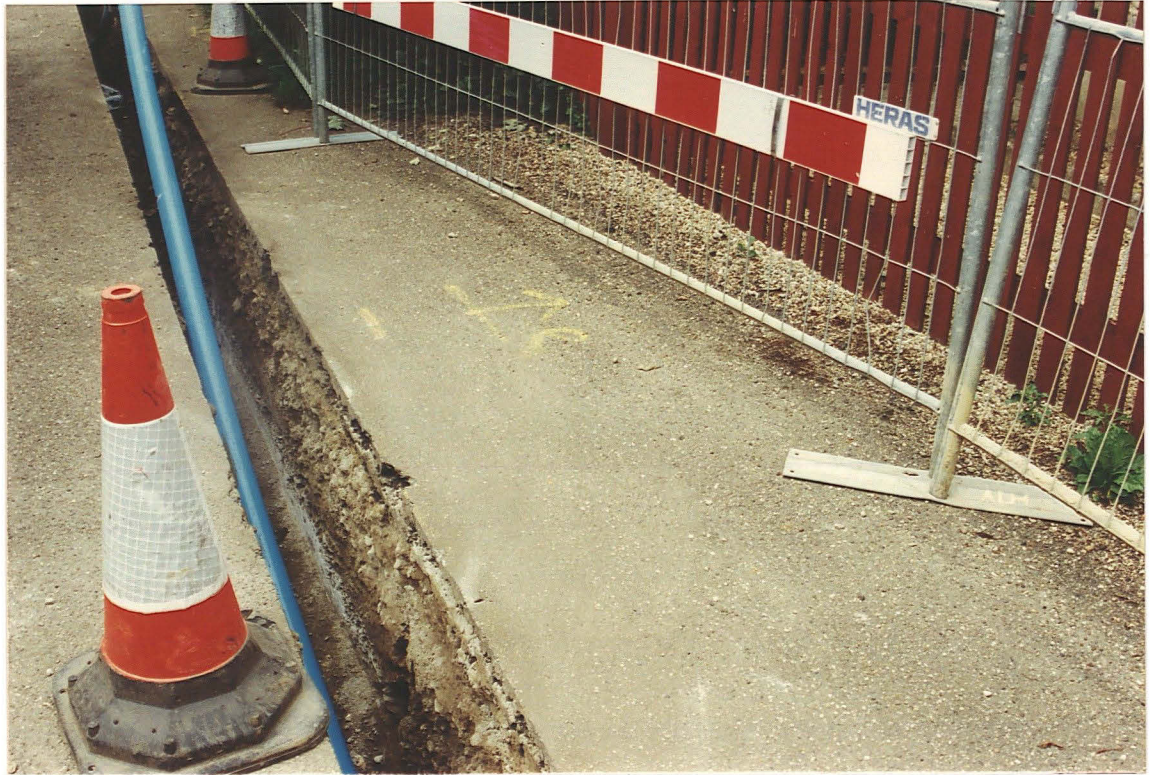
Pl. 3 Position of bedrock ridge 3 in base of trench, in front of Blacksmith's Cottage (looking west).
