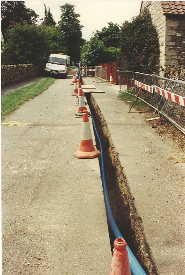
PI. 1 Position of the pipe trench in Church Street, Carlby (looking SW; Blacksmith's Cottage is behind the red fence).
