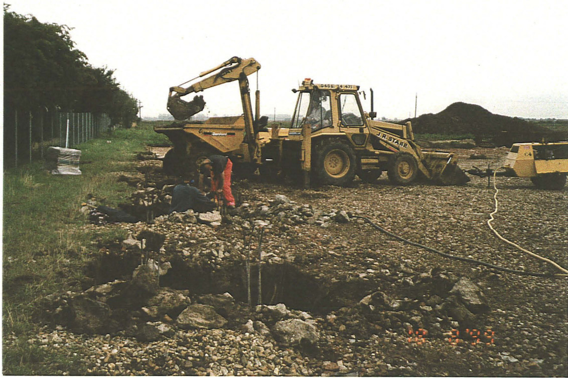
P.3 Working shot of open cut pits on north-east to south-west axis, looking north-east.
