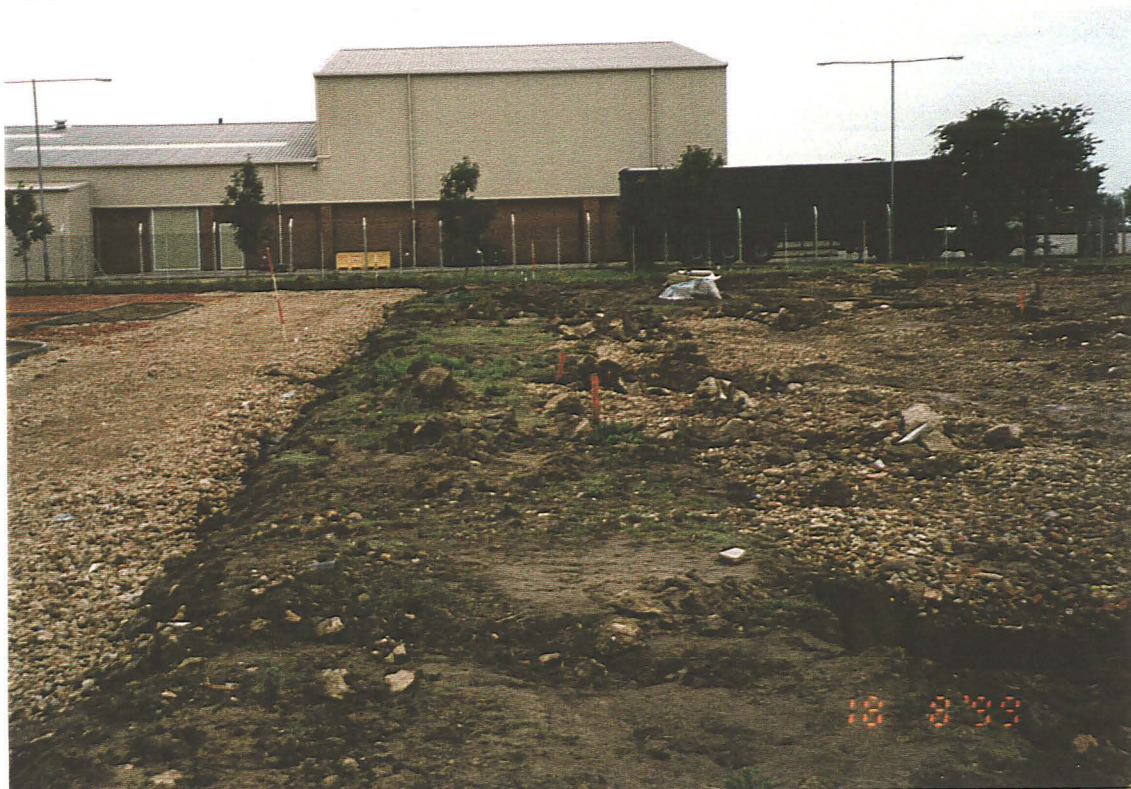
P.1 General view of north-west to south-east line open cut pits, looking north-west.
