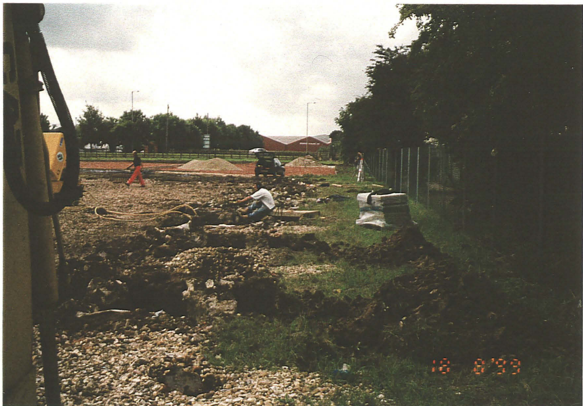
P.4 Working shot of open cut pits on north-east to south-west axis, looking south-west.
