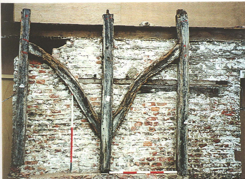
P2. Timbers exposed in south gable
