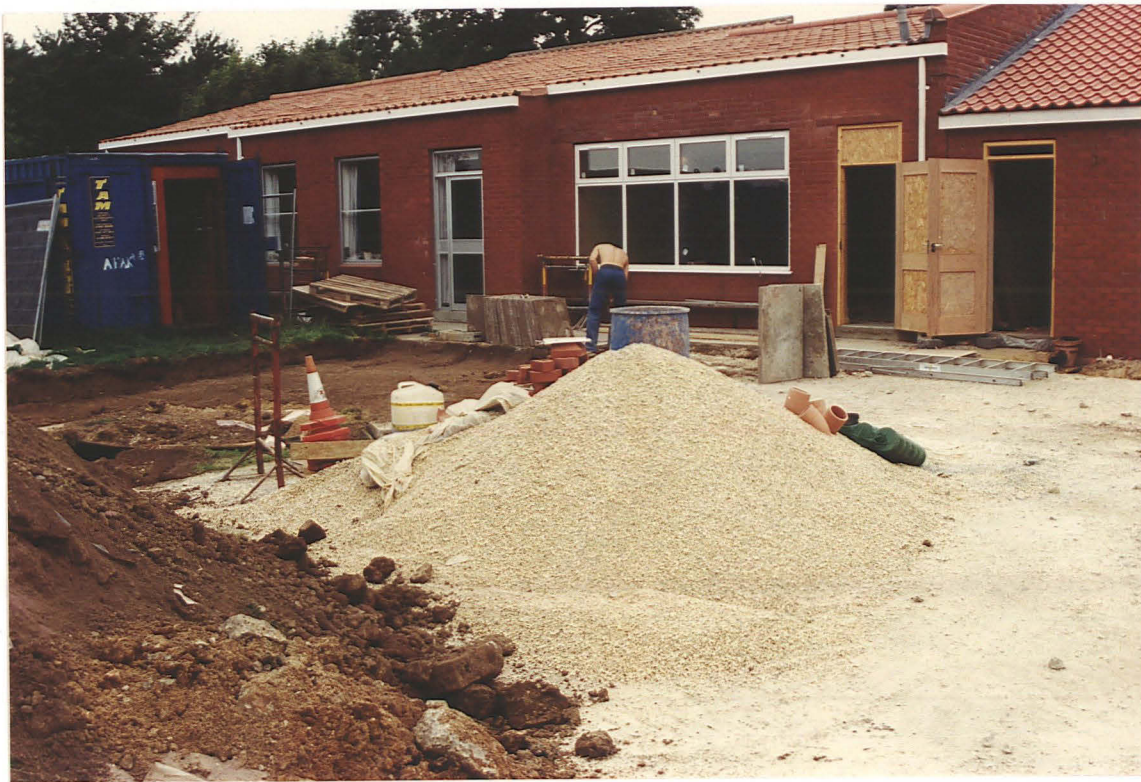
PI. 10 Location of the cleared of topsoil for a new hardplay area, SW of the classrooms. Looking north.
