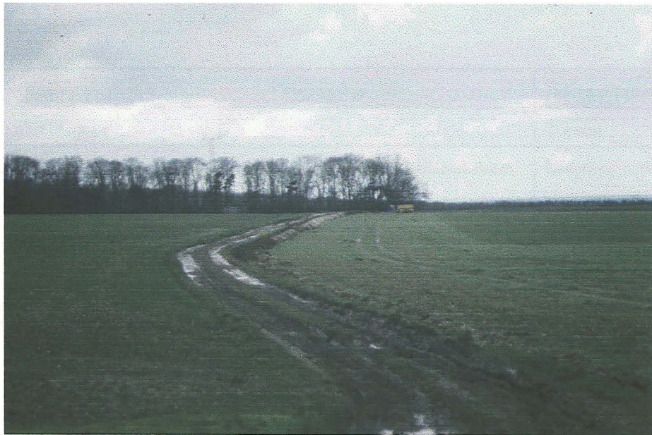
Plate 1 - General view of the cable trench, looking north towards the radio mast (centre)
