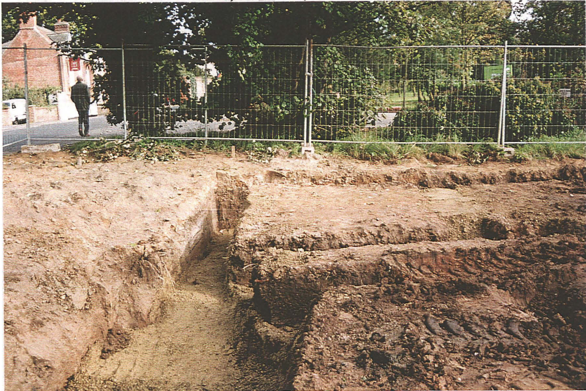
Plate 01: Showing a general shot of Trenches for building construction at Stukely Hall Drive, Holbeach, Lincolnshire.
