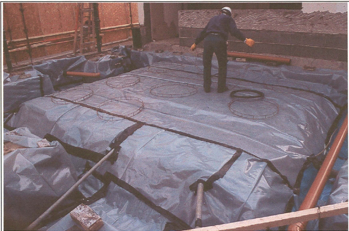
Plate 11: West side of information centre, looking northeast. In order to protect the archaeology exposed but not further investigated during the construction works, a protective sheet was positioned in the trenches.
