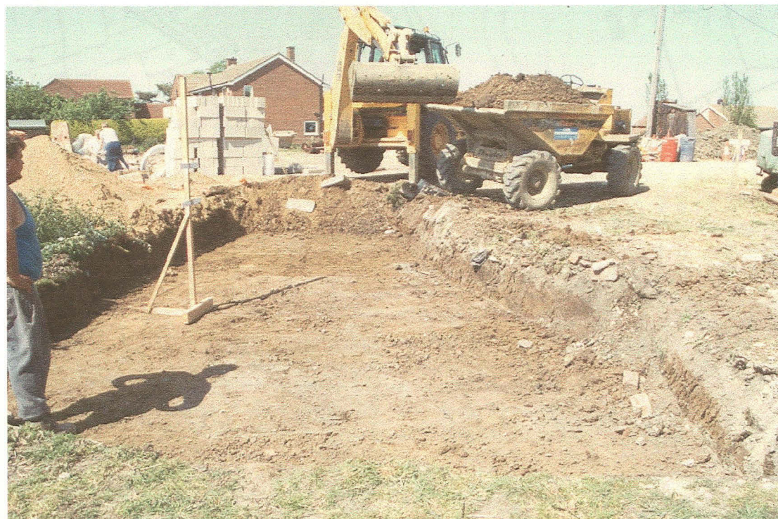
Plate 2: General view of access road (west end), with stripping in progress - looking north
