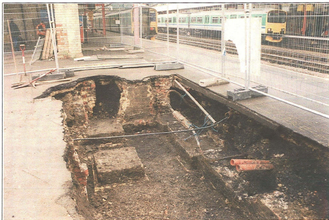
Plate I: General view of the trench located on the southern platform (looking east). Note the many platform-supporting walls and, in the centre of the picture, the four squared pads which supported the original footbridge.
