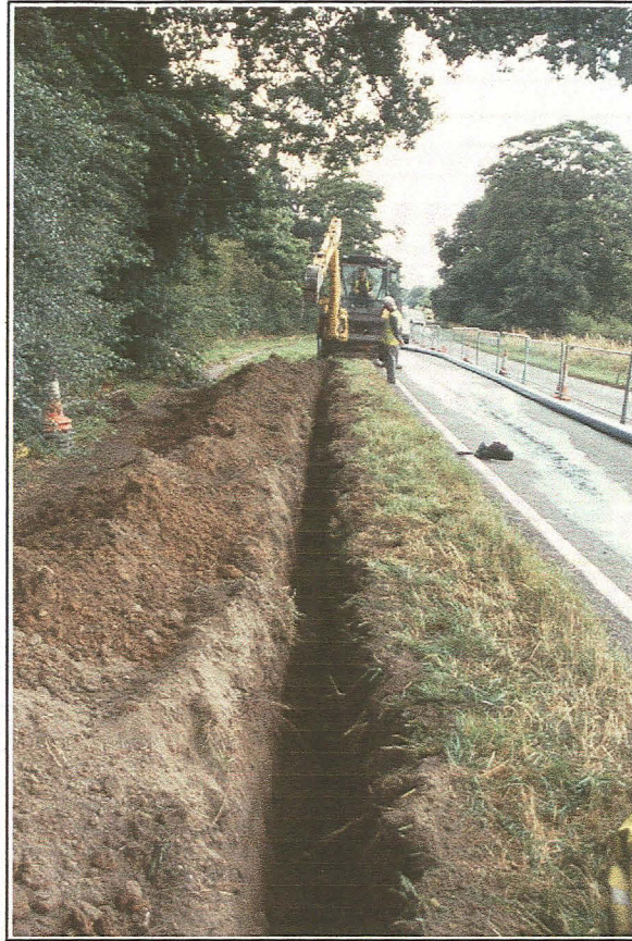
Plate 1: Trenching in progress along north side of A153, Area B - looking east
