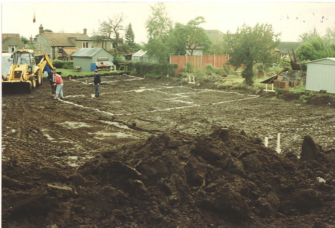
Pl. 1 Site of House Plot 1 and its garage, with the centre of the trench lines marked in white. Looking SE towards Silver Street.
