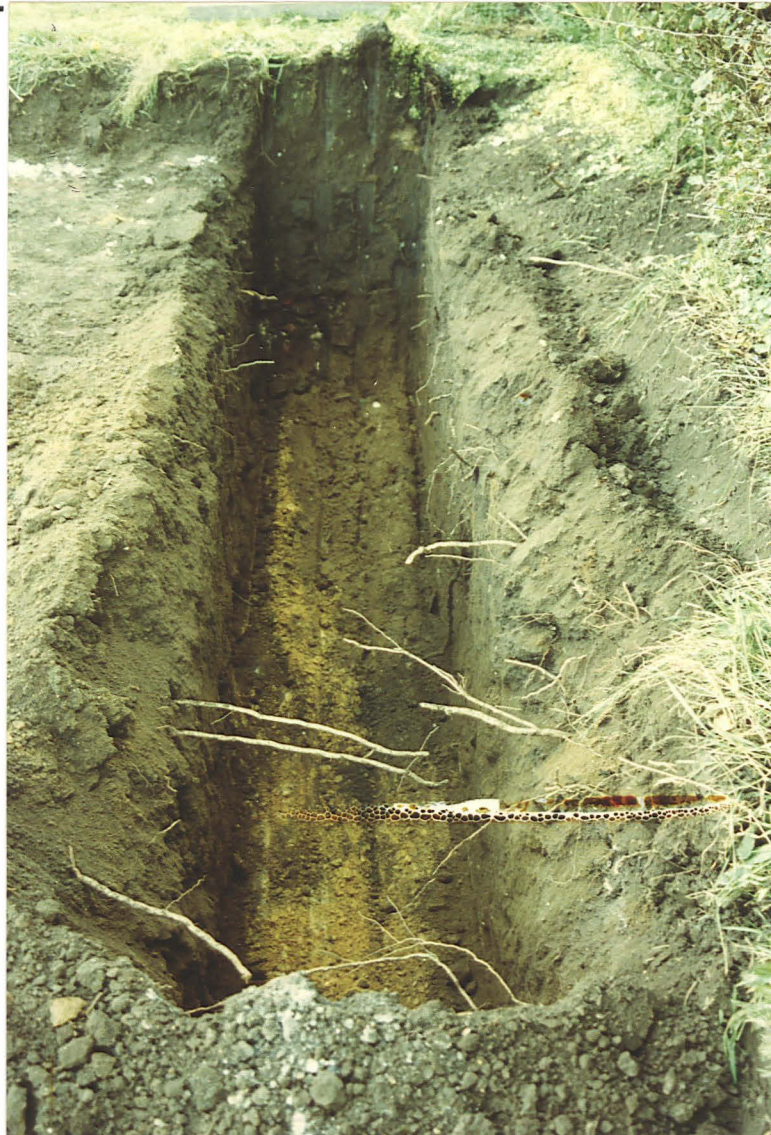
PI. 4 Dark fill of rubbish pit 16 visible contrasting with the yellow brash at the base of the foundation trench, SE corner of the House Plot 1 garage (looking east).
