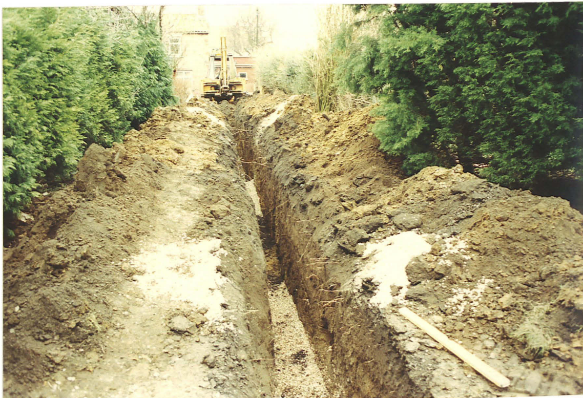
Pl. 6 The service trench, excavated along the access to Silver Street (looking east to the street).
