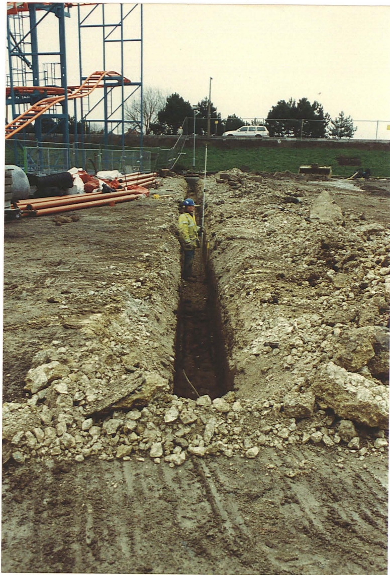
PI. 4 Drain trench along the northern side of the site (looking east).
