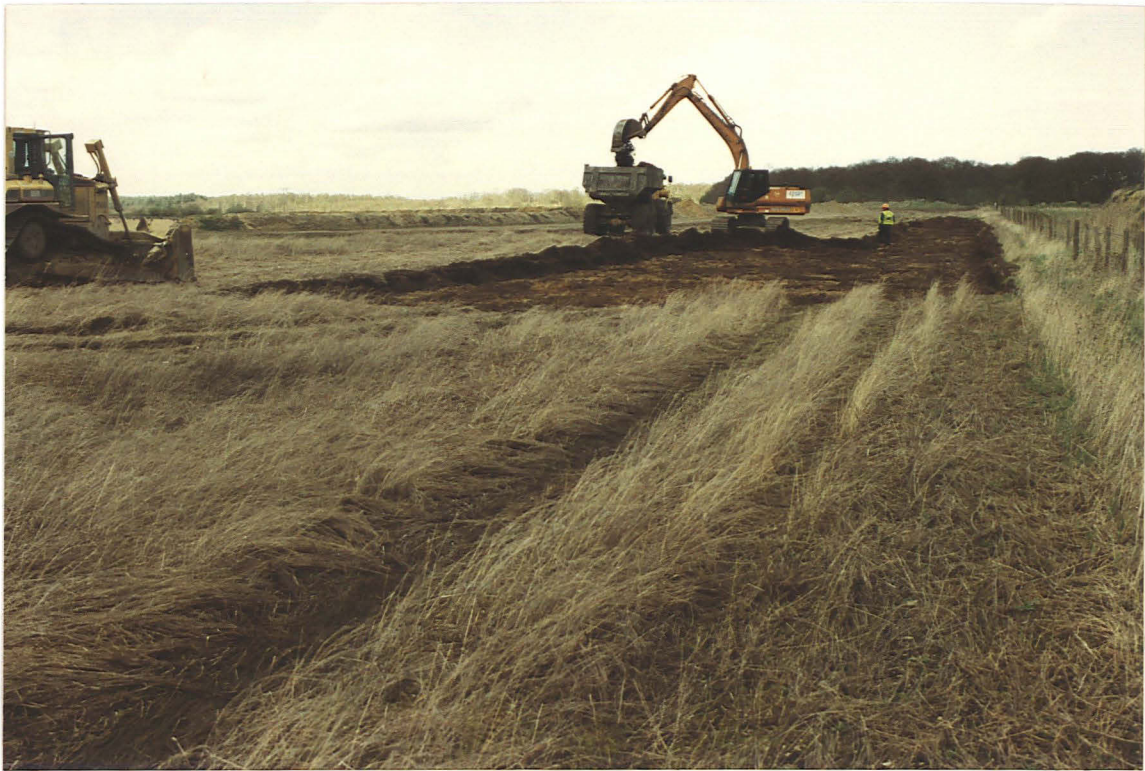
Pl. 1 Topsoil stripping along the southern edge of the Phase 3 area (looking east).
