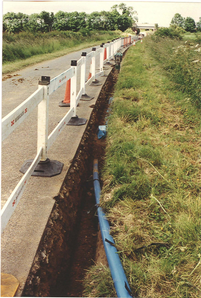
PI. 11 Position of the pipe trench 25, east of the railway bridge on Moor Lane, Branston Moor (looking SW).
