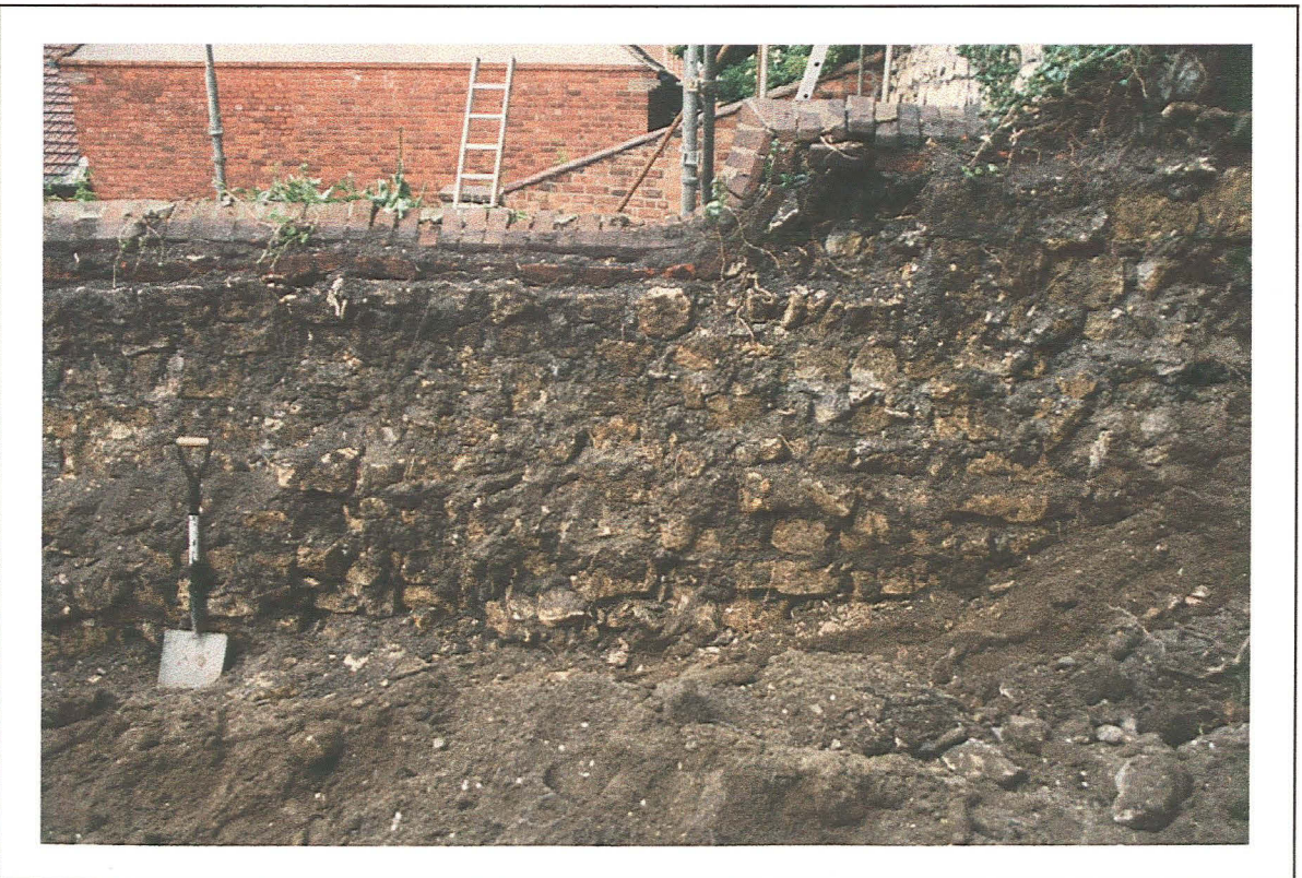
Plate 4: General view of rear of north-south retaining wall, northern end - looking west
