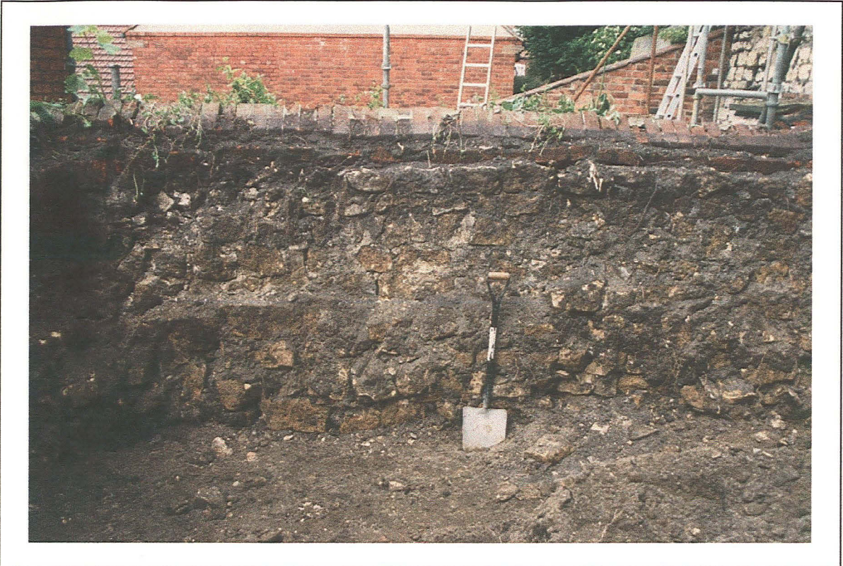
Plate 3: General view of rear of north-south retaining wall, southern end - looking west
