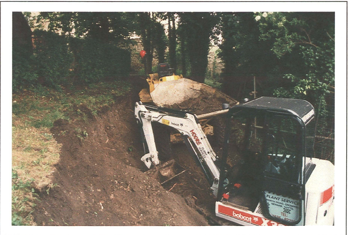
Plate 2: Overall view of dumping material present to rear of retaining wall - looking north-east
