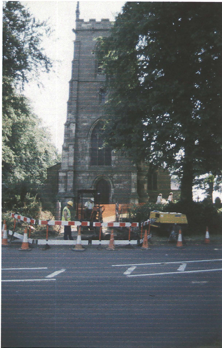
Plate 1 - St. Thomas of Canterbury's church, showing the extent of works, looking east
