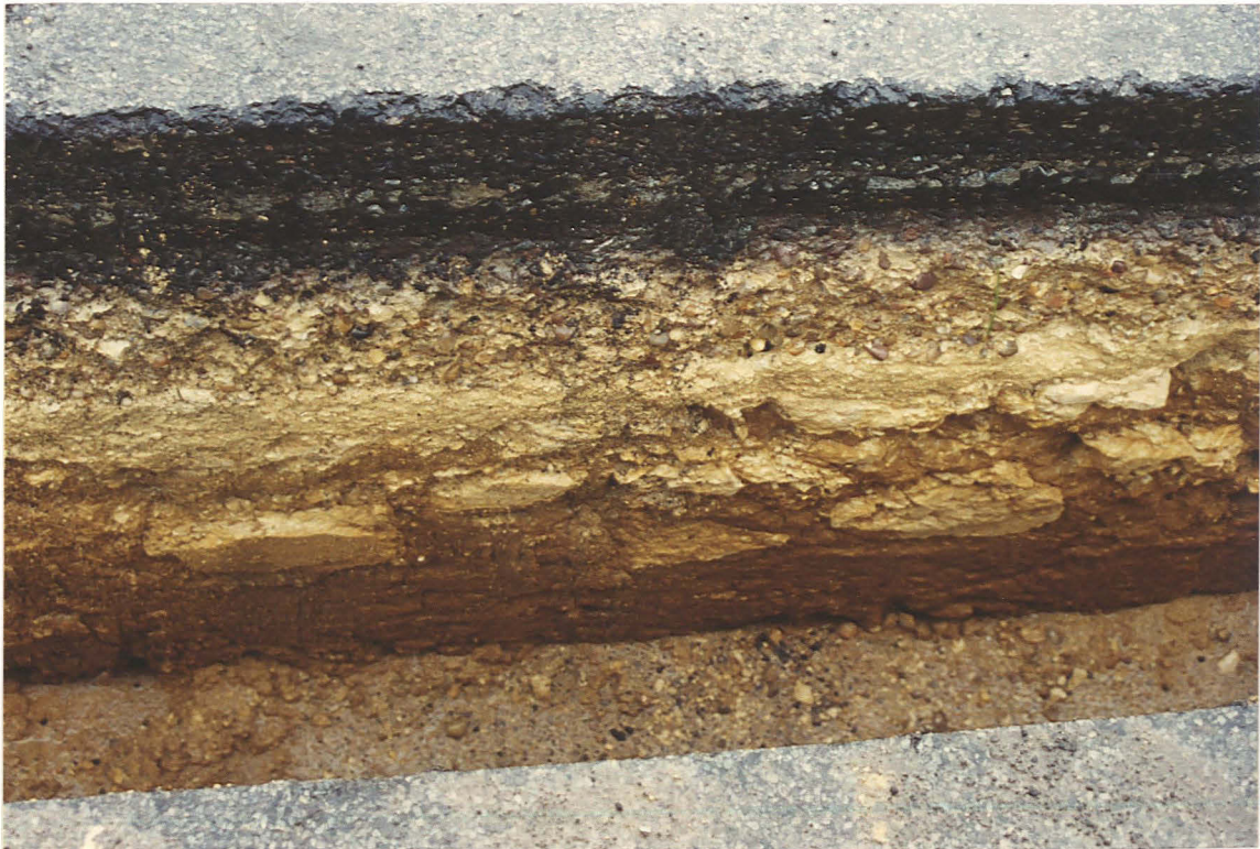
PI. 12 Gravel metalling and limestone block bedding under Grantham Road outside the reservoir 24.
