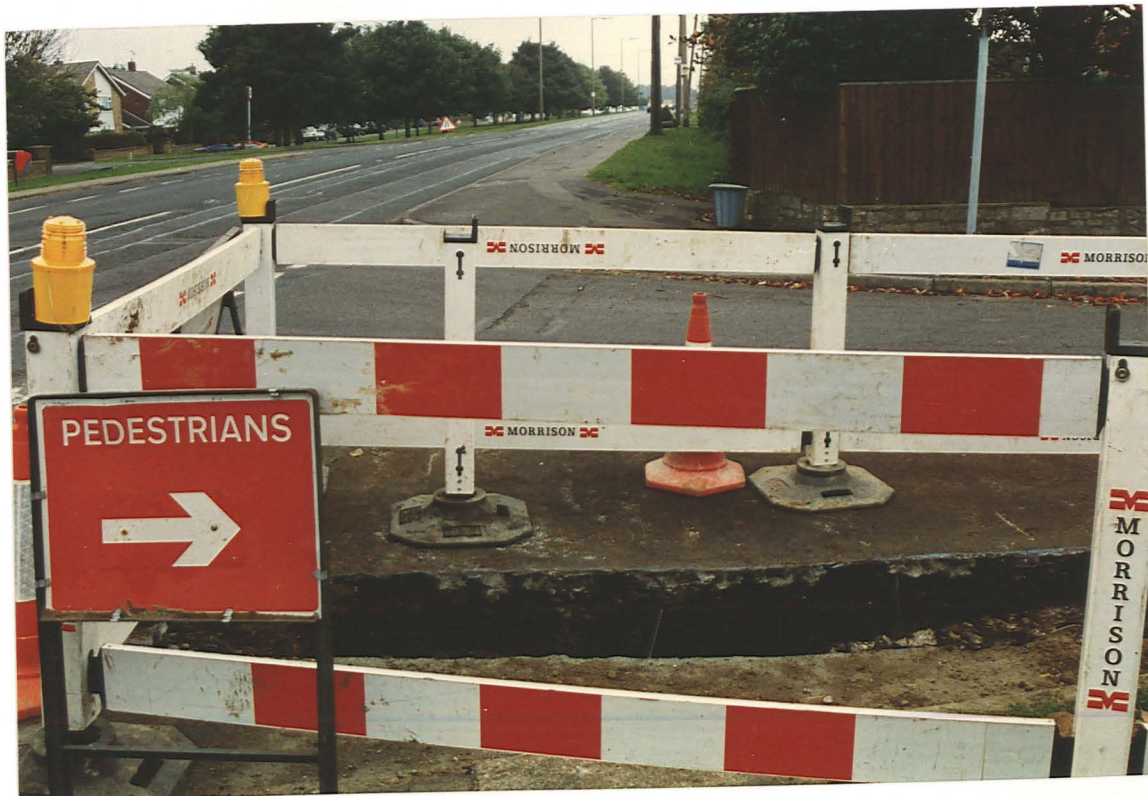
PI. 10 At the junction of Grantham Road and Heath Road 37, evidence for the eastern roadside ditch of Ermine Street was recorded (looking north).
