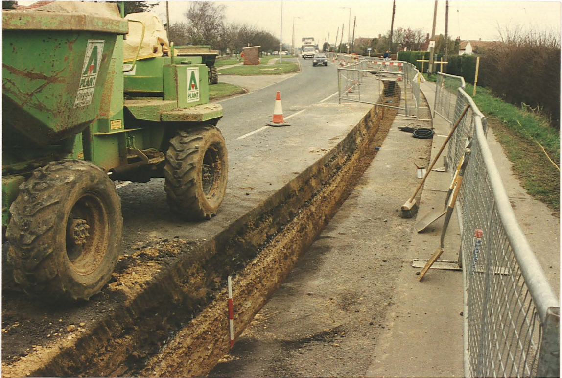
Pl. 5 Gravel metalling thought to represent Ermine Street below Grantham Road at 31 (looking north, scale divisions 0.2m).
